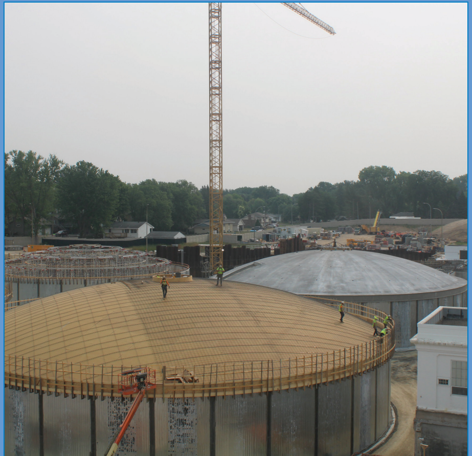
The first cover of the clarifier domes has been laid in concrete on Thursday, June 8, with the dome in the near front slated for the next concrete laying.
