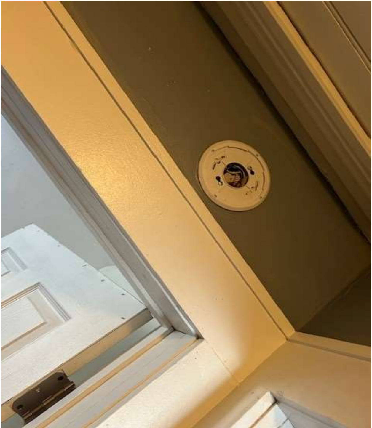
10 shows the missing smoke alarm
