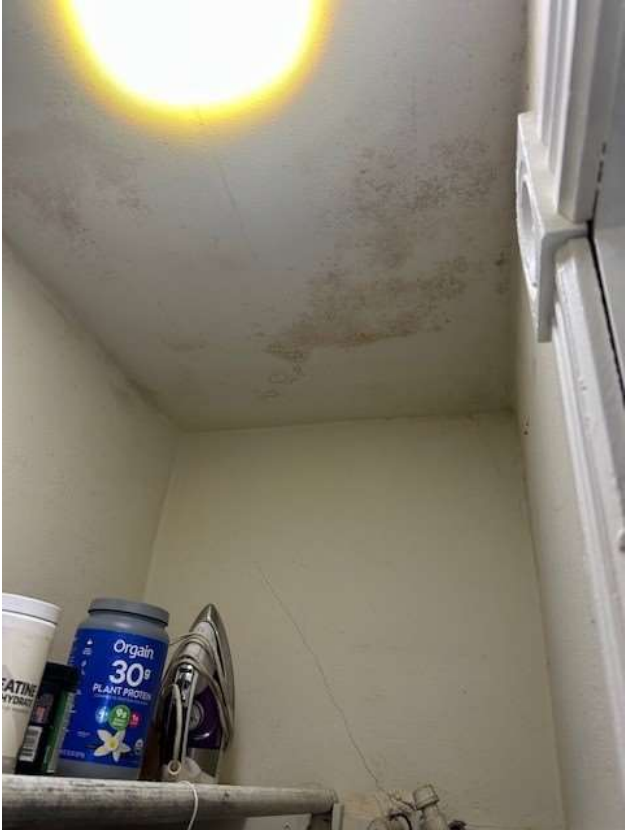
- 9, 11-13 show the water damage and mold like substance in the bedroom and bedroom closet of the upstairs unit.
