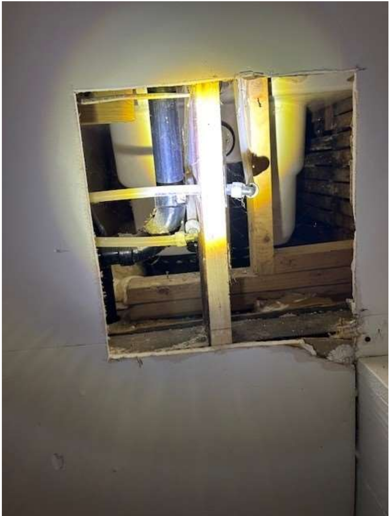
- 8 shows the hole in the wall of the lower units bathroom, in the rear stairwell.
