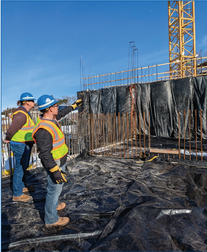
Will Menkhaus, assistant production division manager, points out where the new recarbonation basin will be in the new plant to Aaron Erickson, water utility tech. II, during a tour of the new facilities on March 7.
