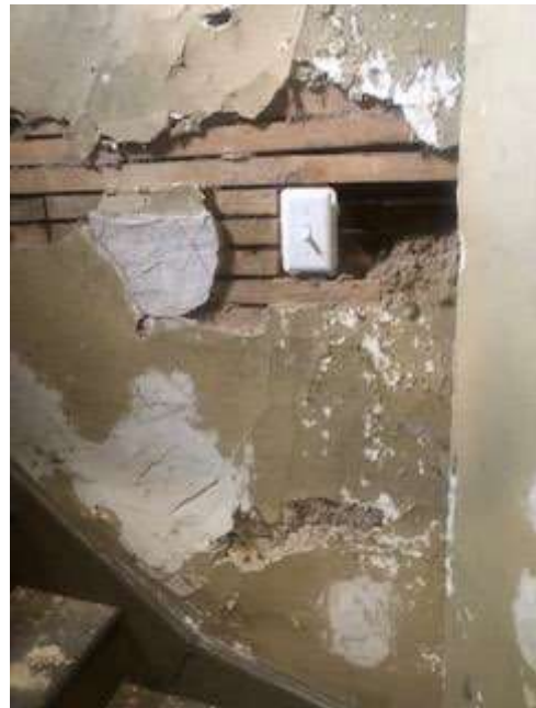
22: Wall deterioration at stairway
