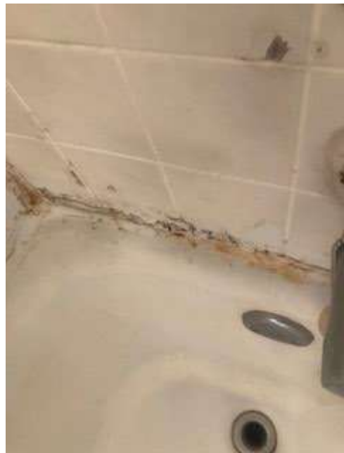
24: Mold and deterioration in unit shower
