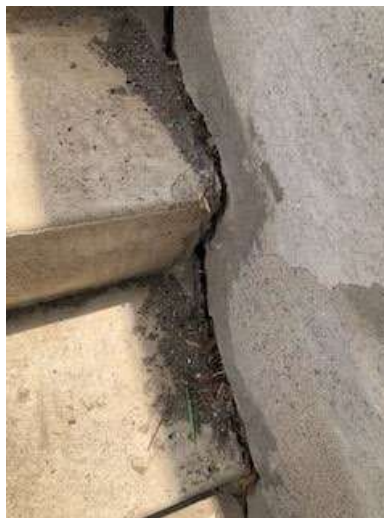
15: Mortar gaps at concrete steps to Unit 5
