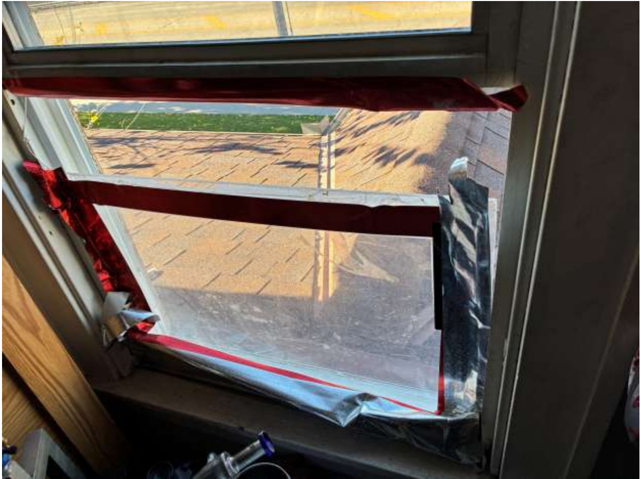
10. close look at bedroom window is not operational and taped up
