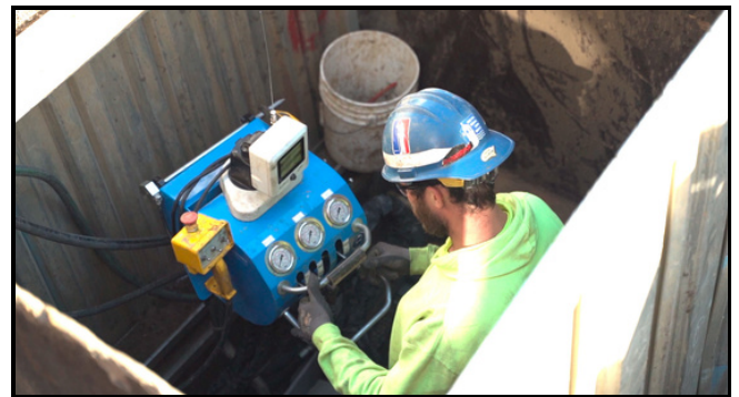
A worker guides horizontal drilling equipment underground to allow for a new copper service line to be pulled through from the house to the street during a lead replacement.
