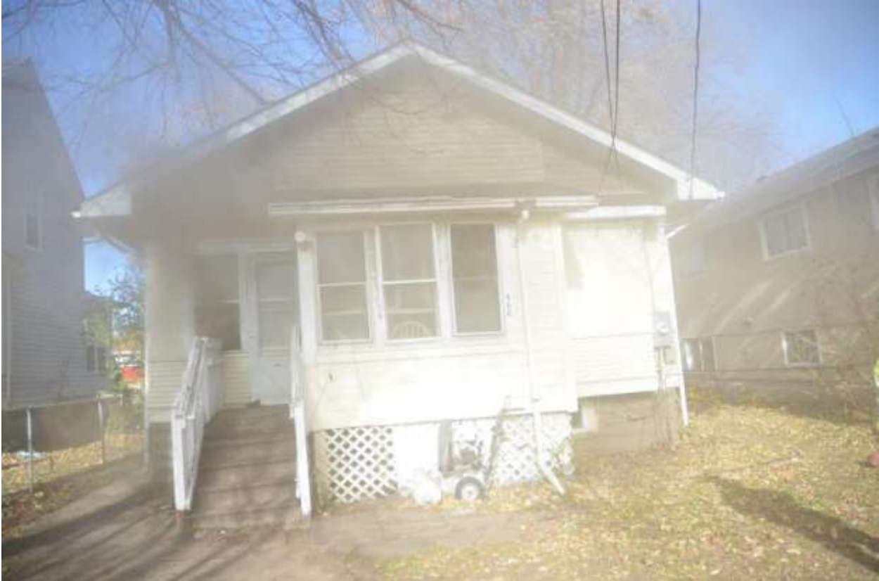
468 Thomas Ave.Fire Dwelling Photos 11-18-23
