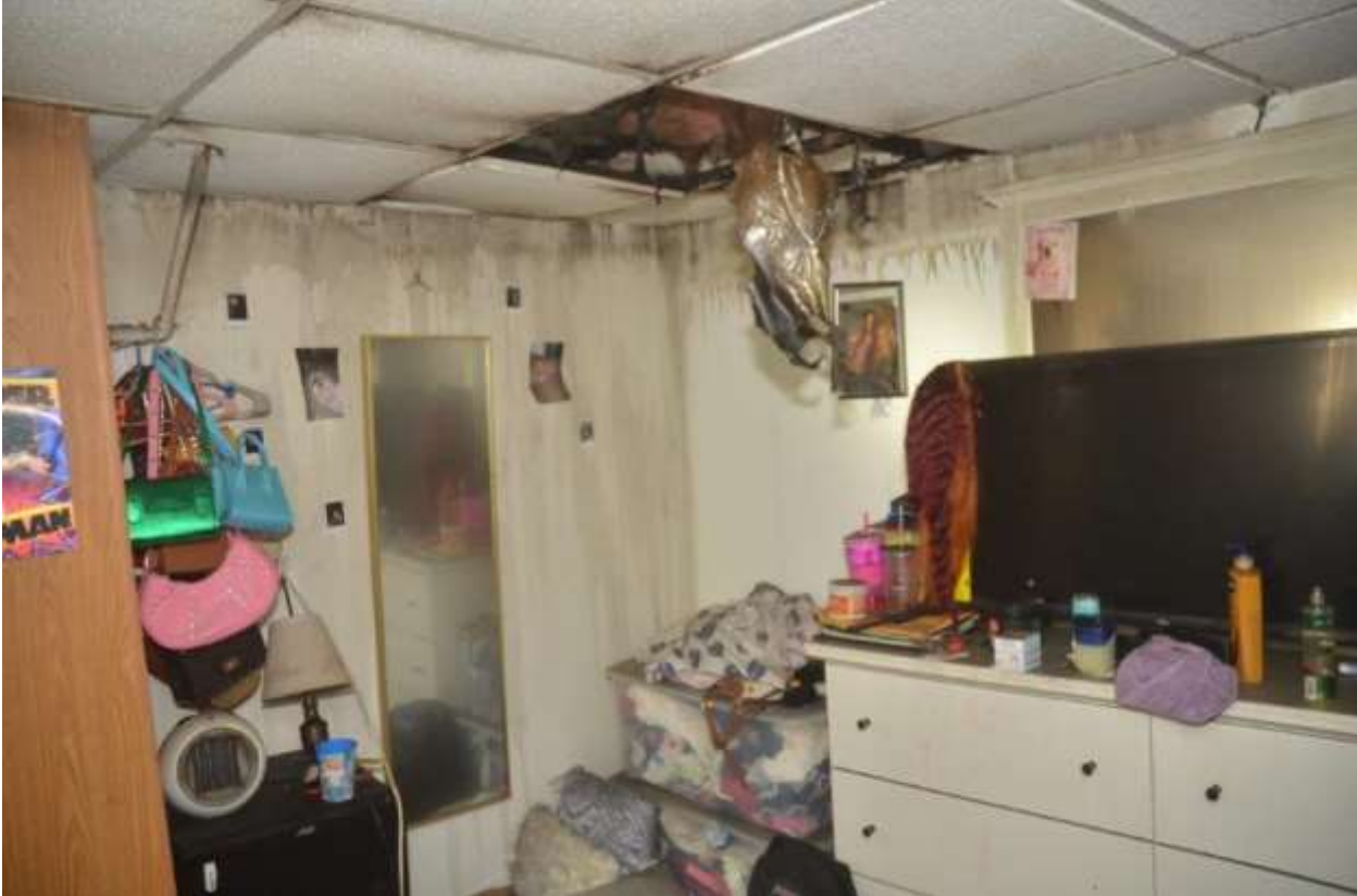
468 Thomas Ave.Fire Dwelling Photos 11-18-23
