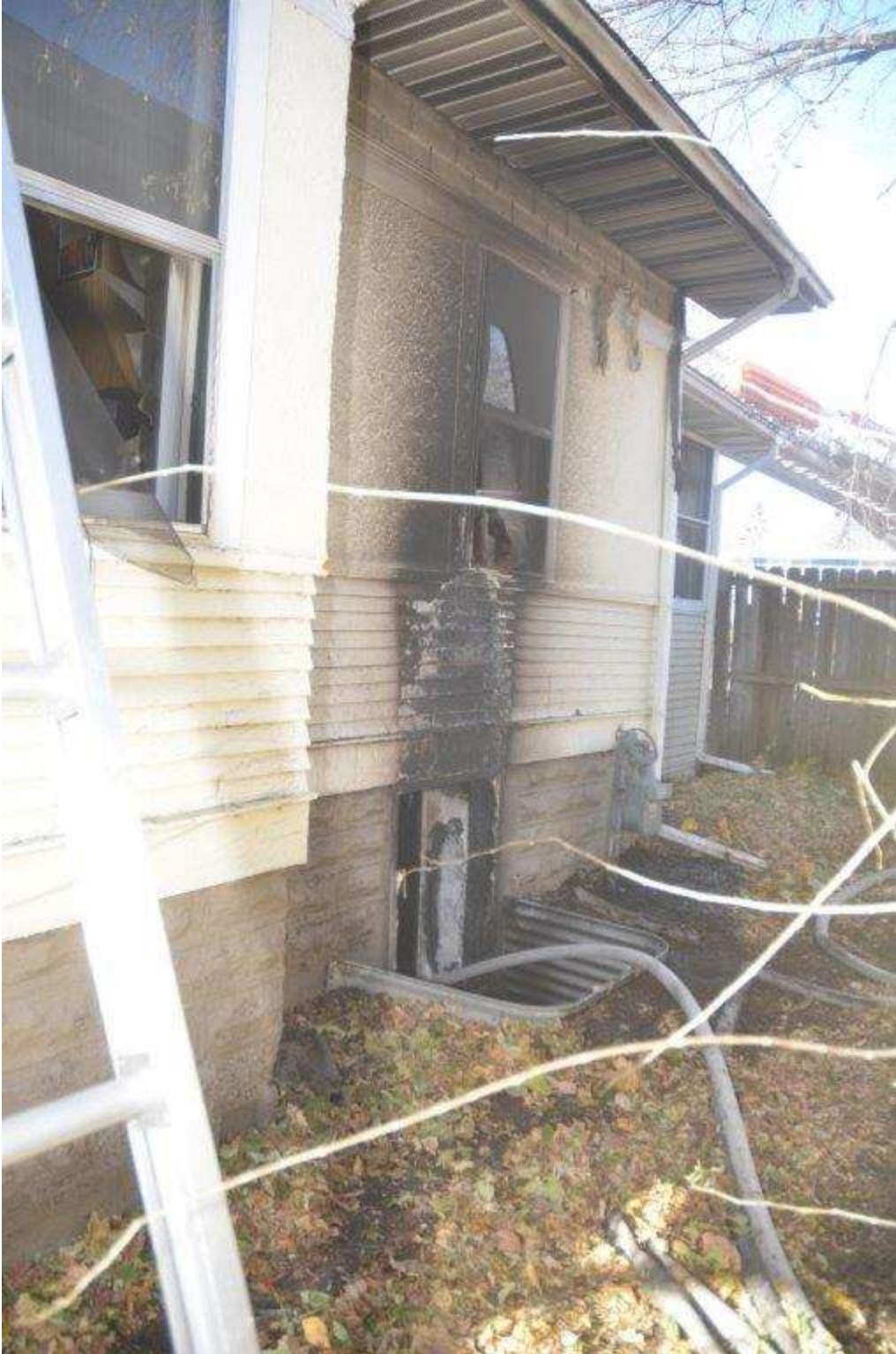
468 Thomas Ave.Fire Dwelling Photos 11-18-23
