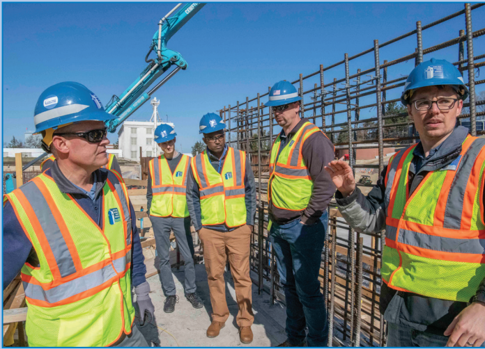
Above, Will Menkhaus, right, gives a tour of the work site of the treatment plant project on April 25.
