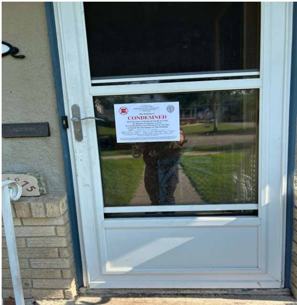
1875 Nebraska Ave E. Condemned placard
