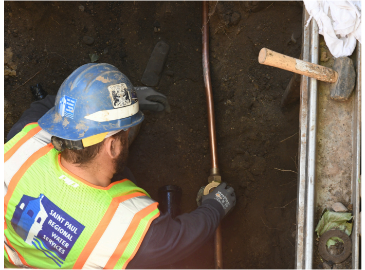
A worker connects a copper service line from private property to the copper service line in right of way.
