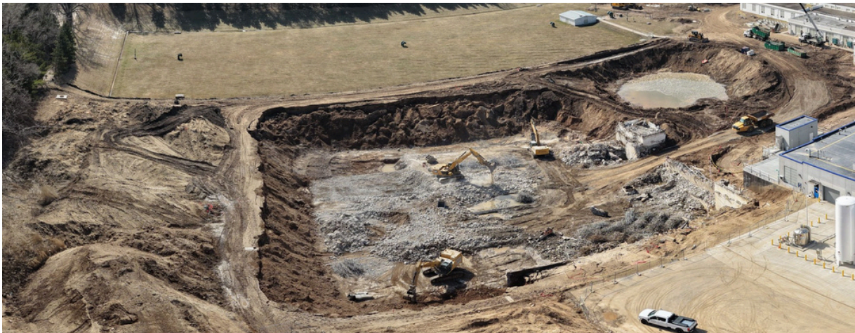
Clarifiers 2 - 5 along with floc 3 and the recarb basins being demoed in late March.
