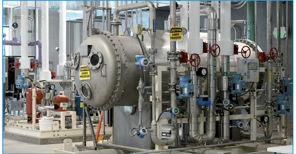
An ozonation tank in the ozone room in the new plant.
