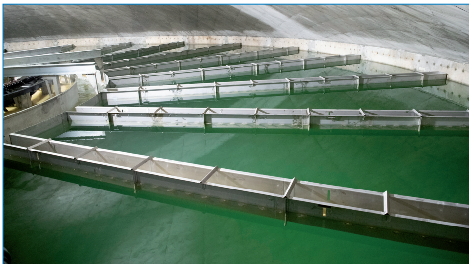
The new clarifiers are online and have been operating since July 8 in the new treatment plant.
