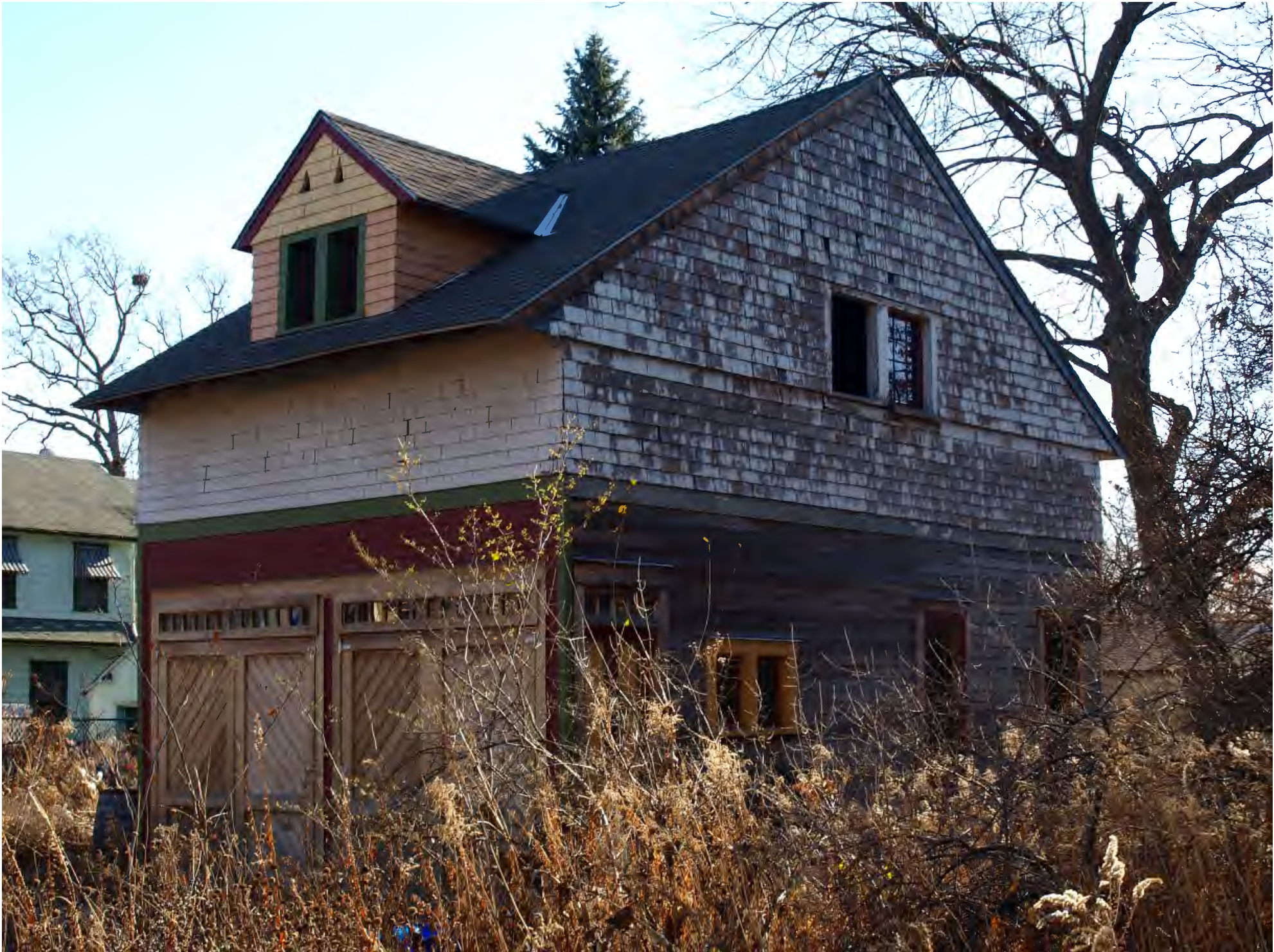
Dwight and Clara Watson House_0010 barn viewed from northwest, north and west elevations, camera facing southeast
