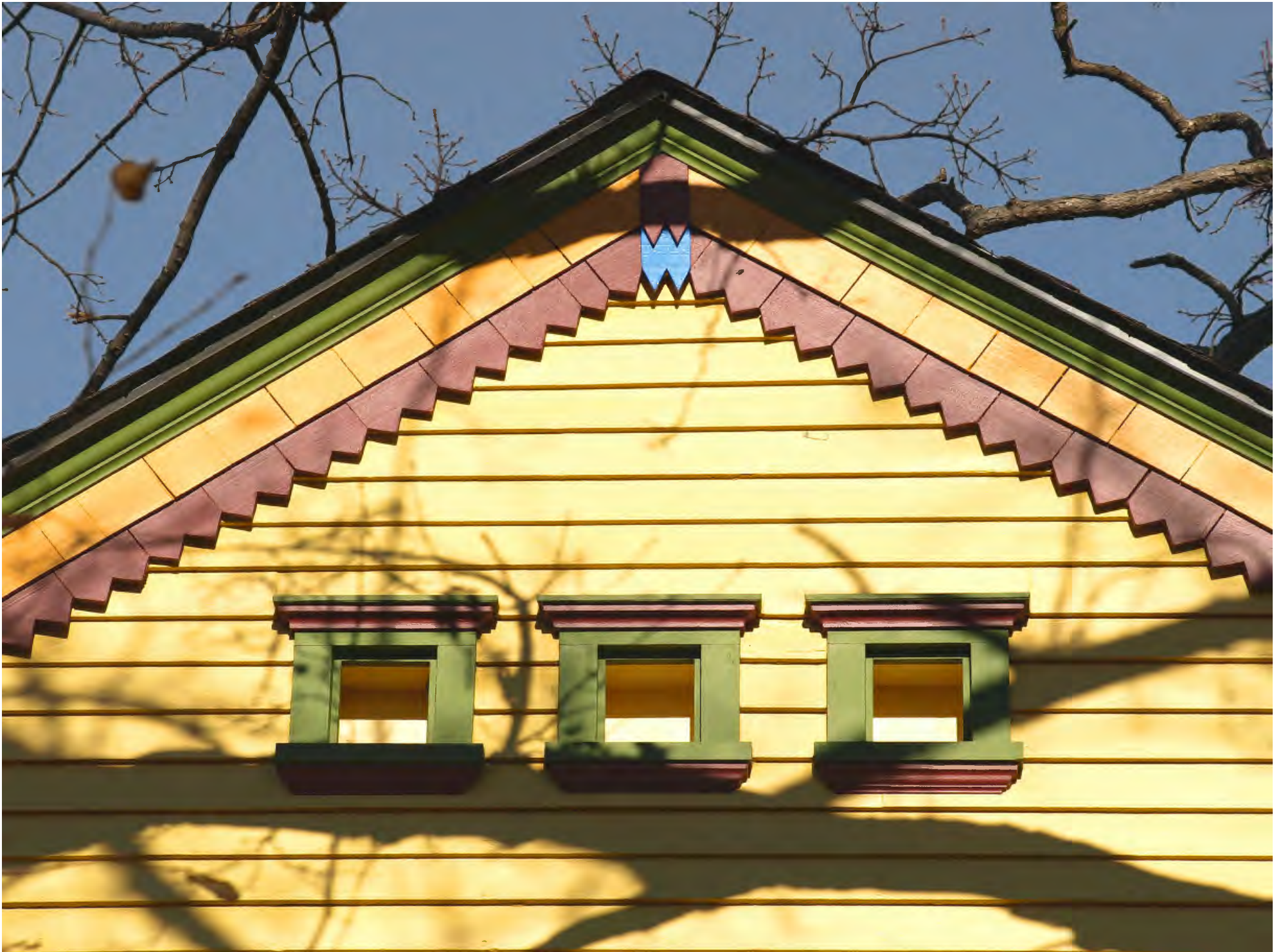
Dwight and Clara Watson House_000 house detail viewed from south, south elevation, camera facing north
