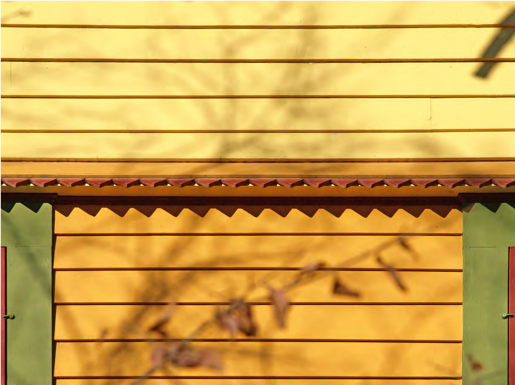
Dwight and Clara Watson House_000 house detail viewed from south, south elevation, camera facing north
