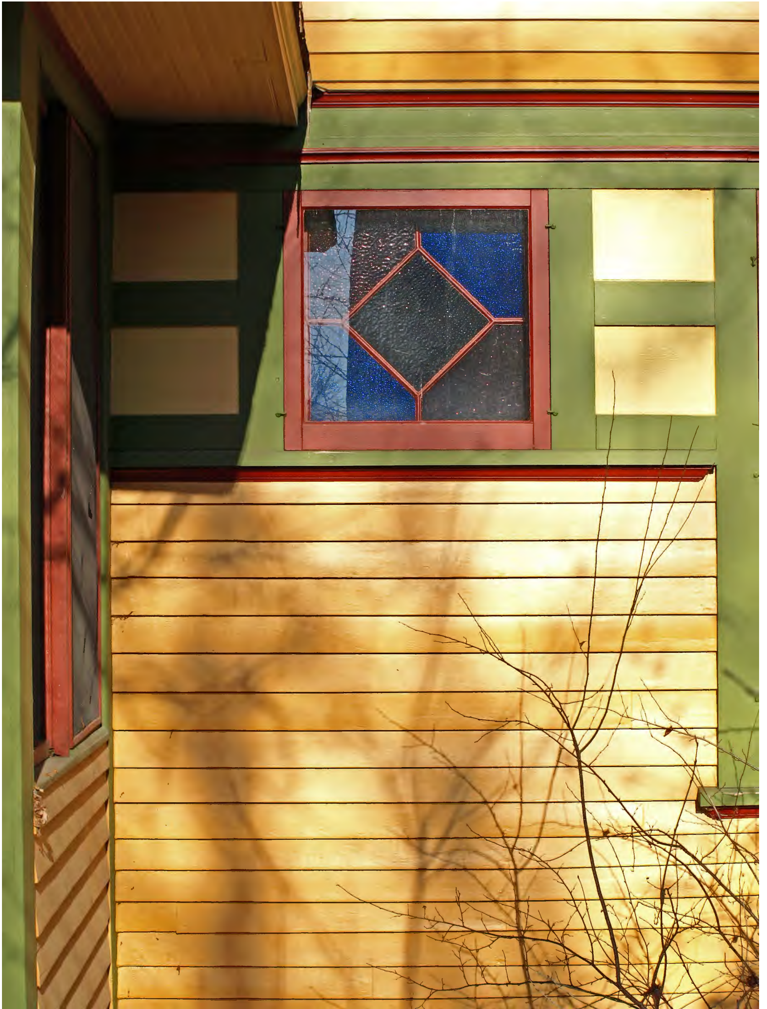
Dwight and Clara Watson House_000 house detail viewed from south, south elevation, camera facing north
