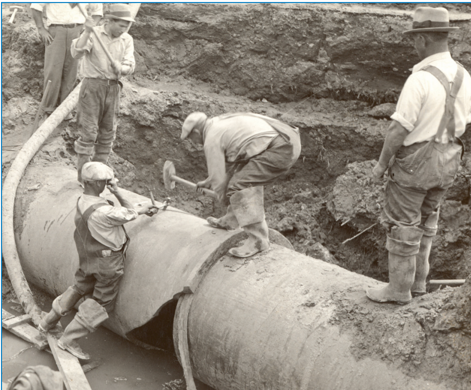
Workers make repairs on a 36-inch water-main in this undated photo. These images are part of research being done to make a
