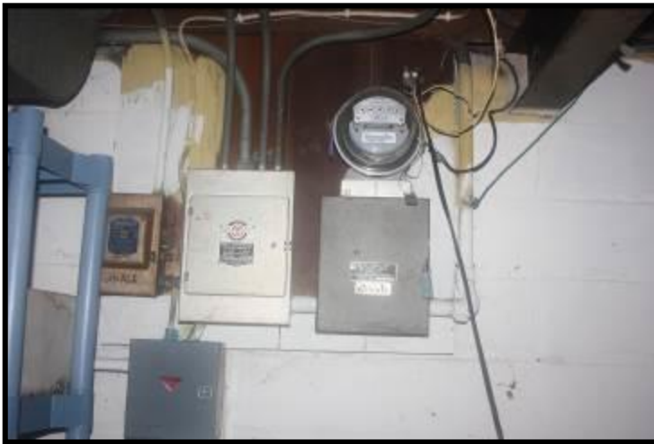
Original electrical infrastructure: 30 Amp
