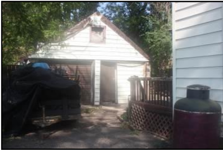
Garage in poor condition needs to be removed
