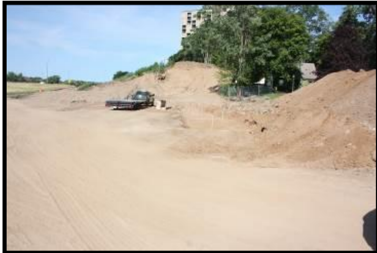
View west along the Metro Gold Line BRT now under construction Just south of subject along existing R/W
