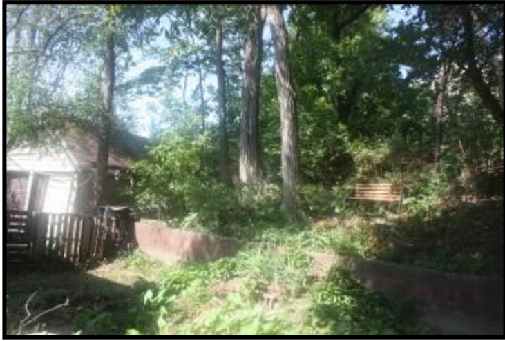
Rotted roof; garage built into hillside to west
