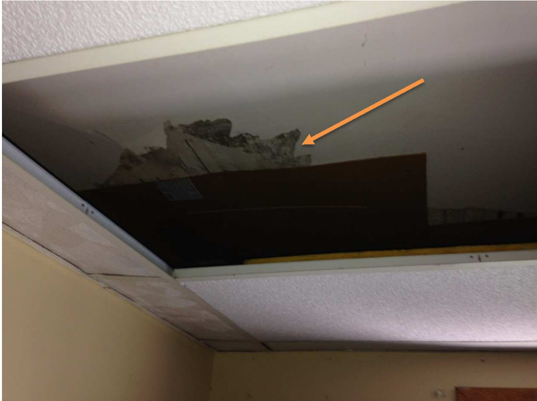
Picture 4 – Water Damage to 2 nd Floor Ceiling
