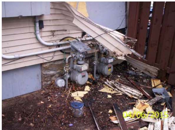
Gas meters locked off
