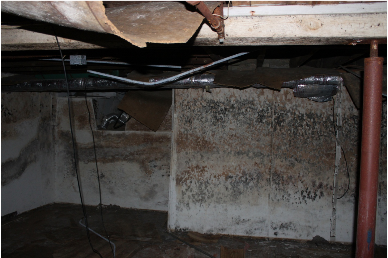
Basement conditions (above), exposed section of original Eastlake style balusters and newel posts (below left), and mortise & tenon detail of upstairs door.
