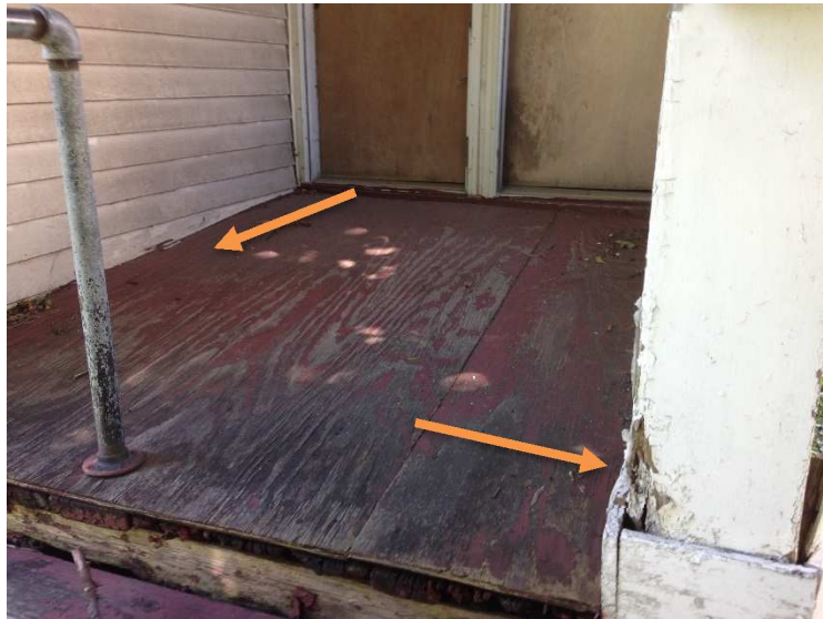
Picture 5 – Front Porch Deterioration and Slope
