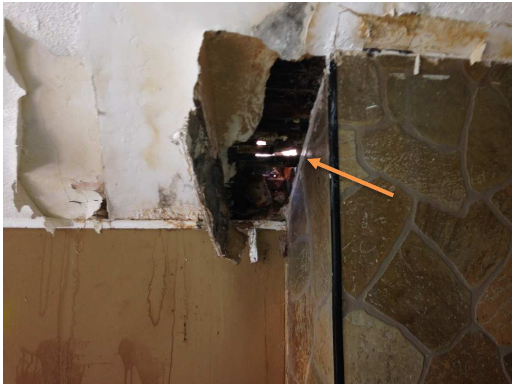
Picture 11 – Rot Through Roof
