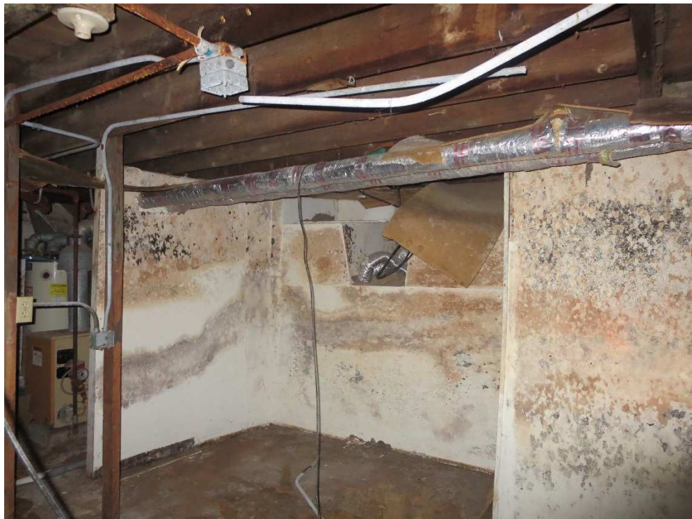
Picture 18 – Mold in Basement
