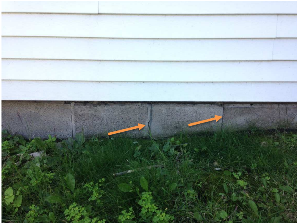
Picture 14 – No Mortar Between CMU Units
