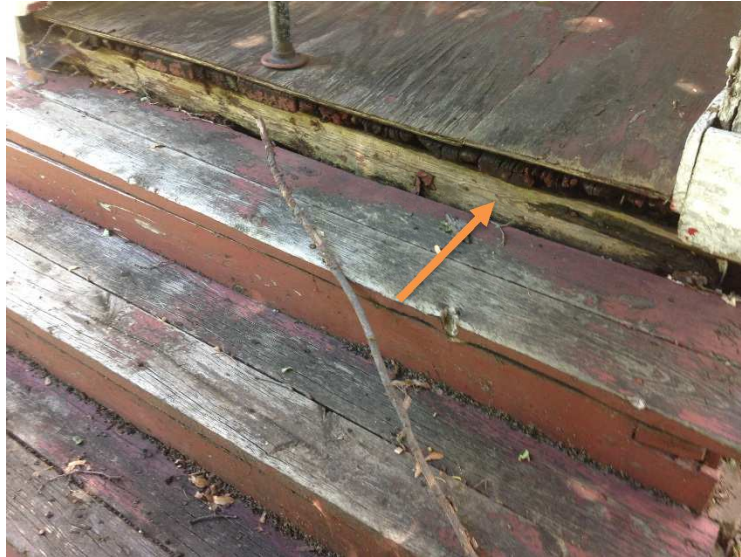
Picture 4 – Front Porch Deterioration
