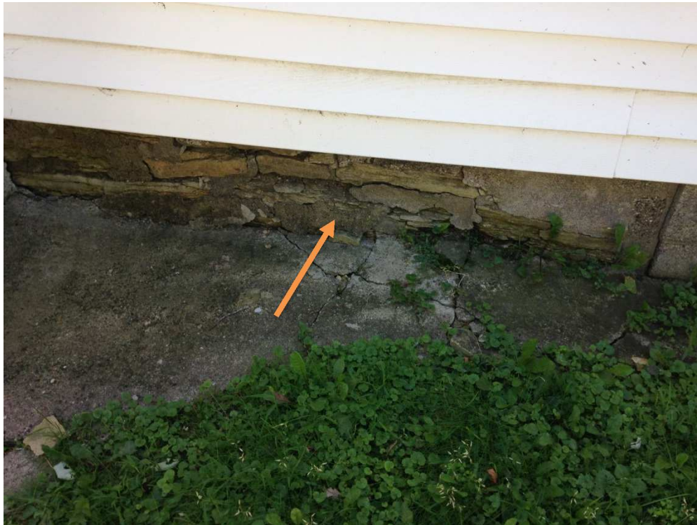
Picture 12 – Foundation Deterioration
