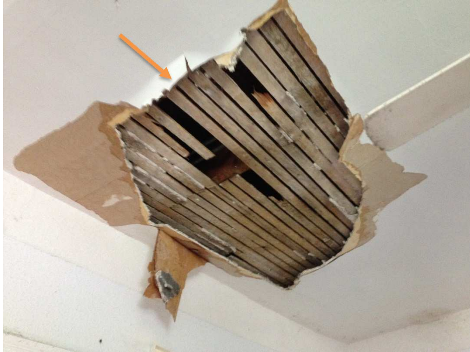
Picture 17 –Damage to Ceiling
