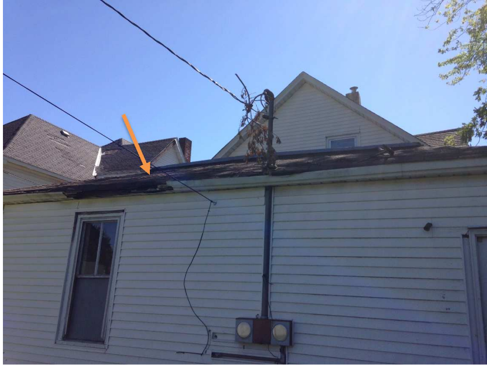
Picture 10 – Rot At Back Roof
