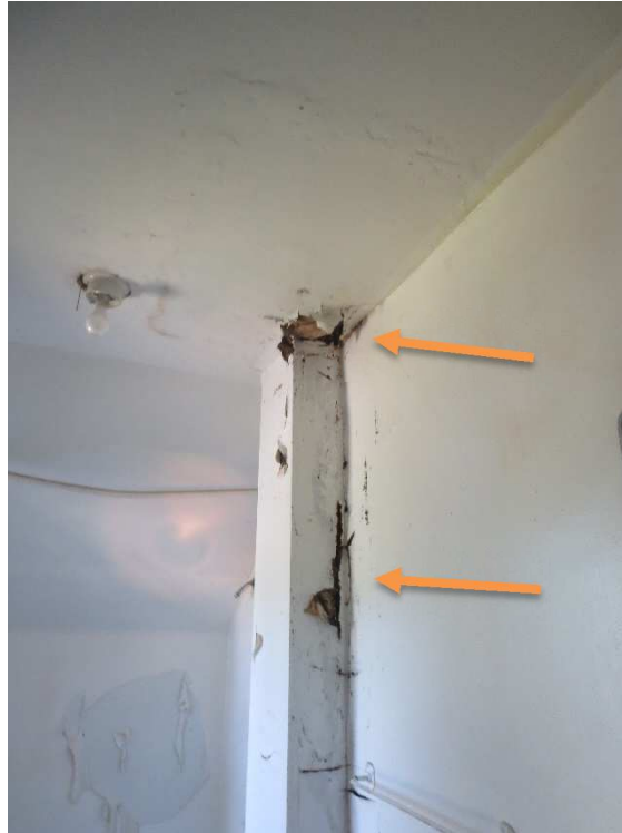
Picture 16 – Water Damage to Column
