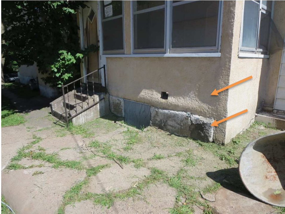
Picture 7 – Water Damage at Southern Foundation Wall
