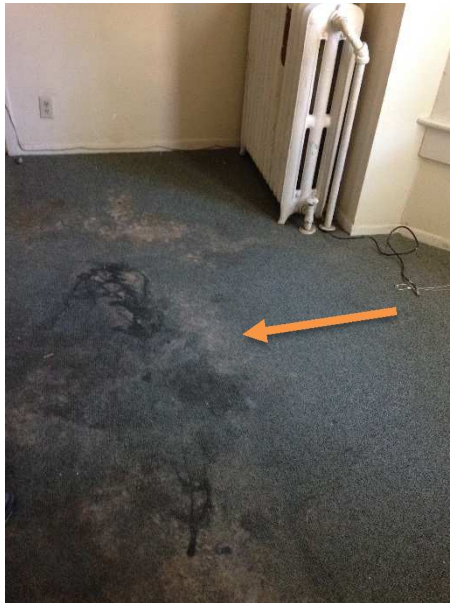
Picture 8 – Water Damage in 2 nd Floor
