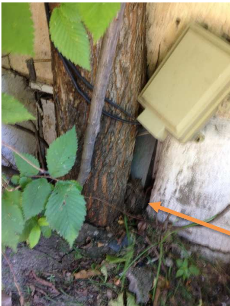
Picture 6 – Tree Growing Next to House
