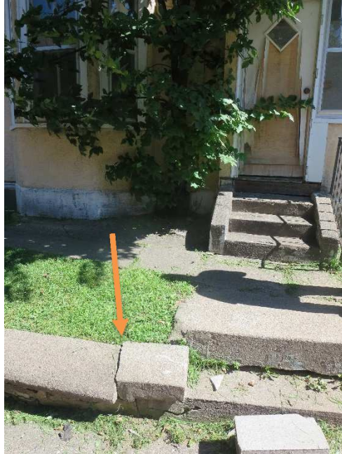
Picture 4 – Crack at South Retaining Wall
