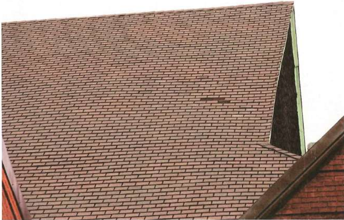
Figure 7 Detail of current portion of south side eastern end of main roof showing missing shingles 7/27/15
