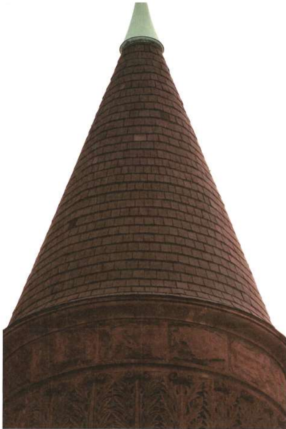
Figure 11 Detail view of turret on northwest corner showing missing shingles 7/27/15
