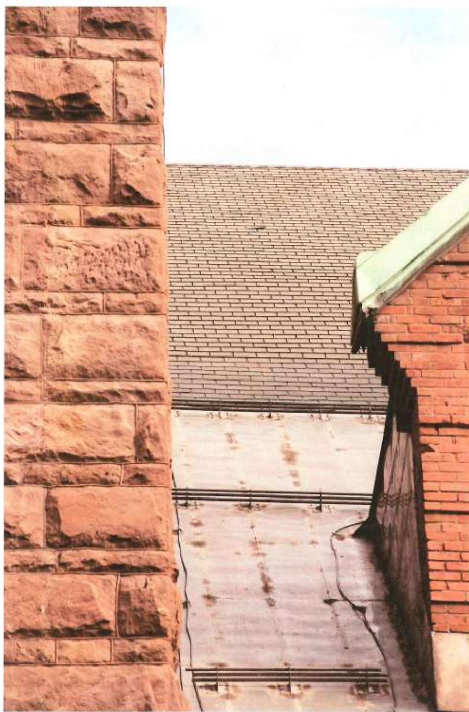
Figure 8 Detail view of south side main roof by bell tower showing missing shingles 7/27/15
