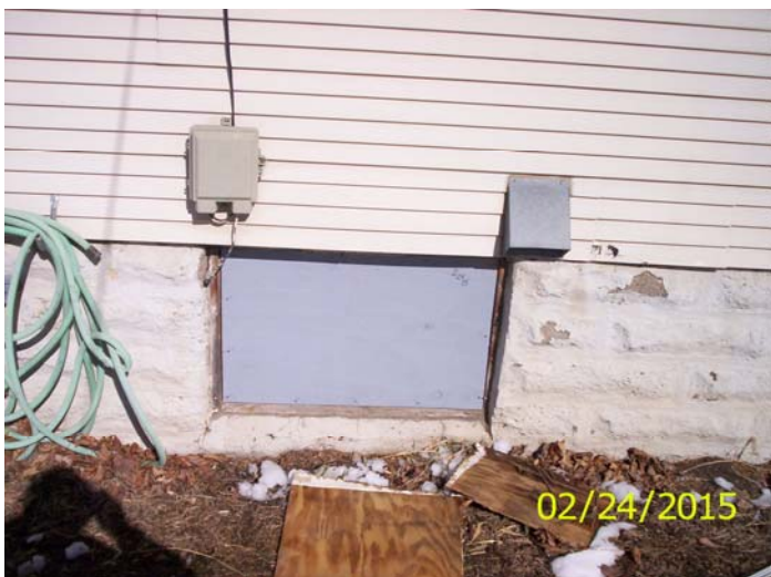
Boarded south side basement window
