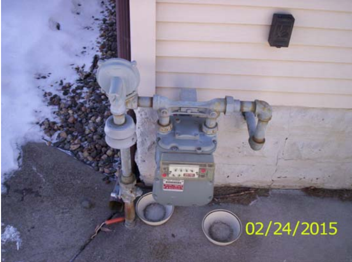
Locked gas meter
