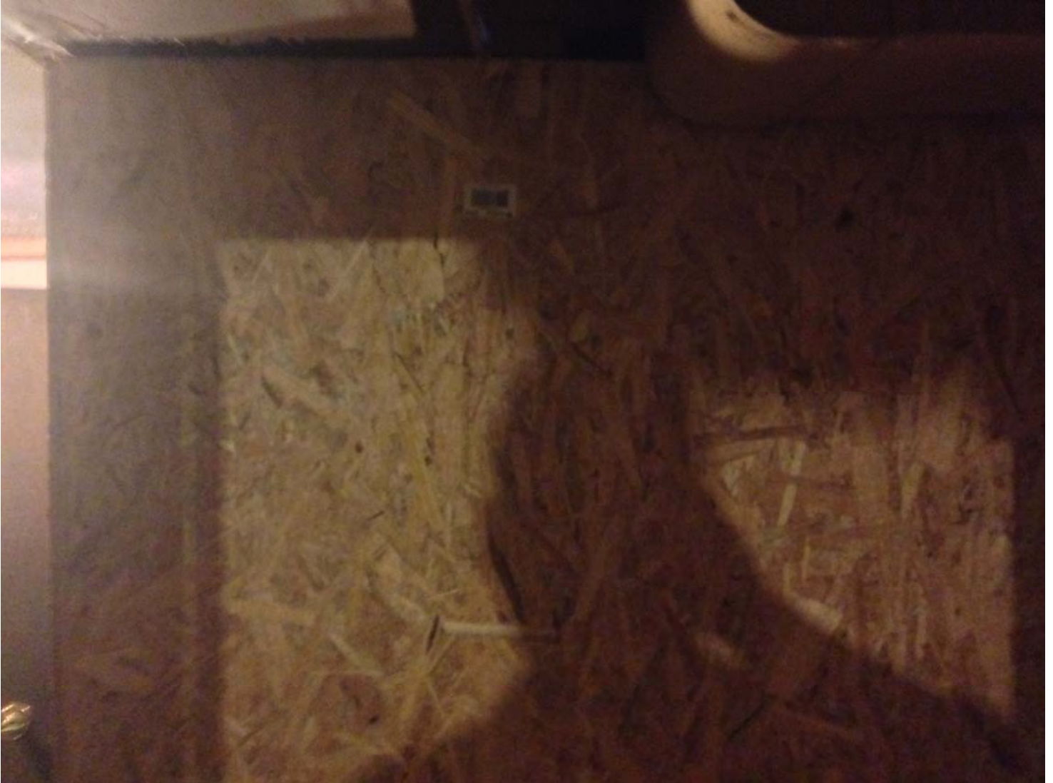
¼ Newly installed since last inspection OSB used to enclose unapproved basement bathroom.
