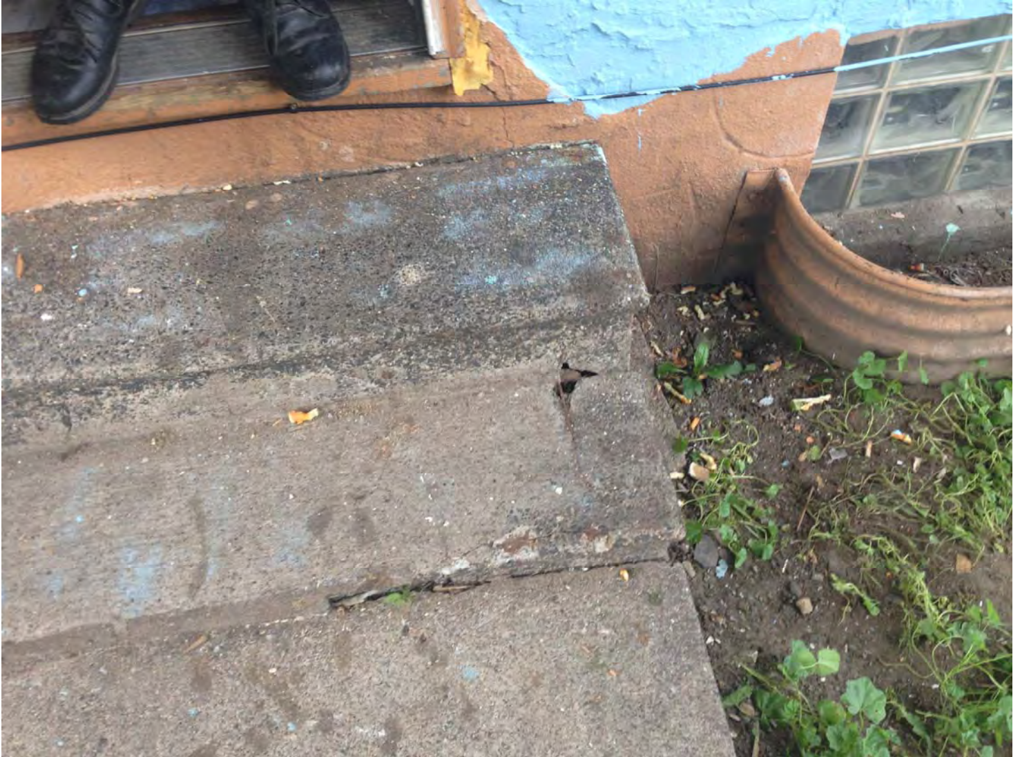
Deteriorated front steps, exposed rebar
