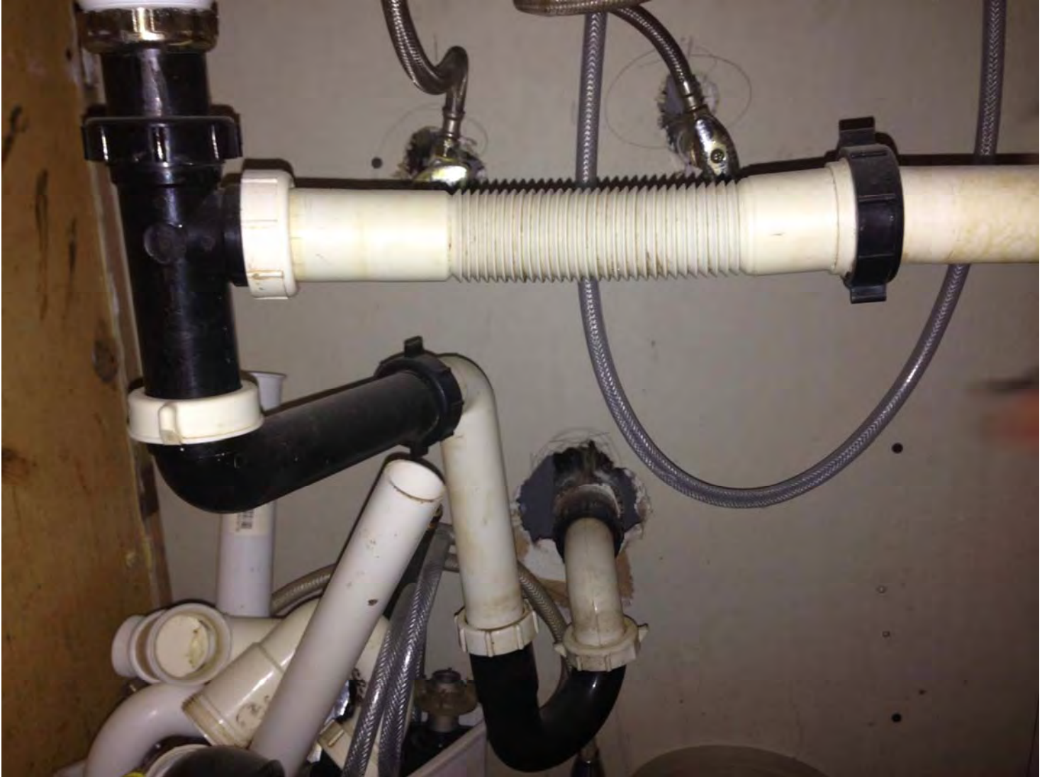
Plumbing improperly installed and incorrect materials installed without permit
