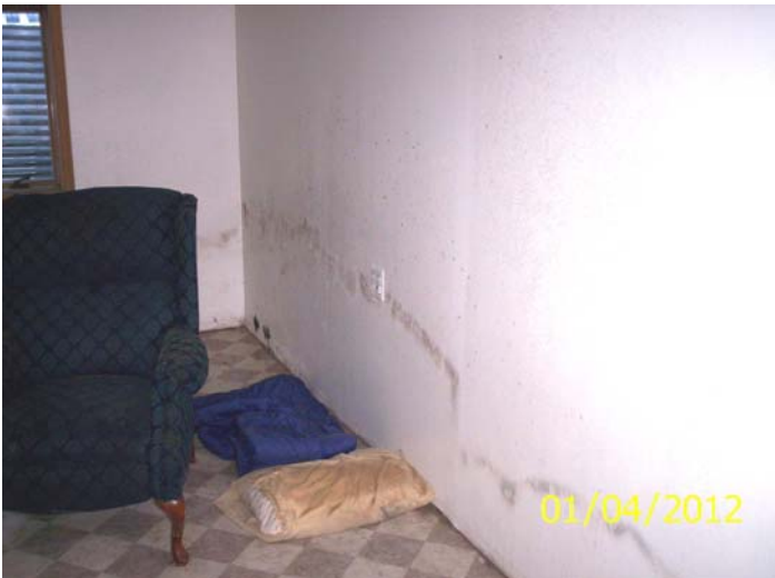
Mold in basement
