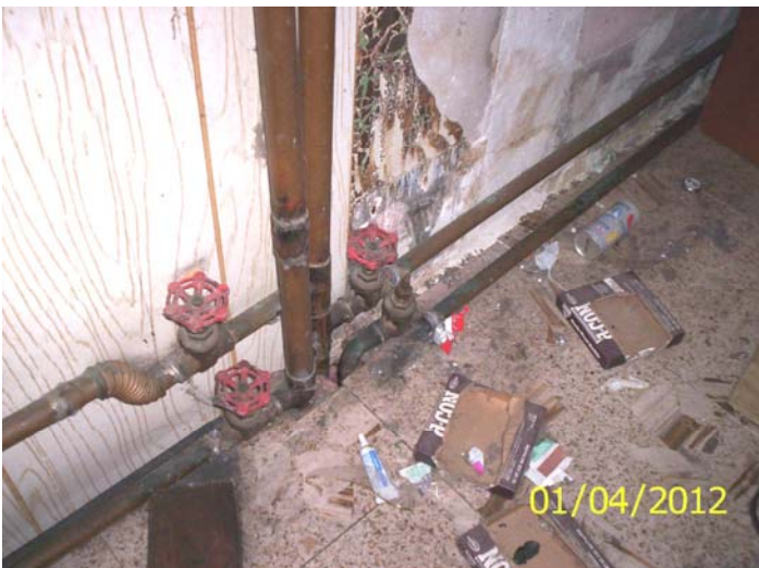
Water damaged wall, open water line, mold
