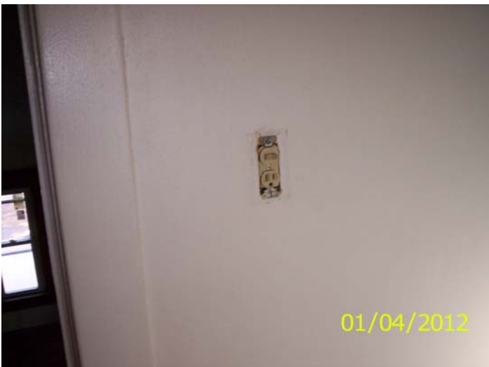
Missing cover plate; exposed wiring
