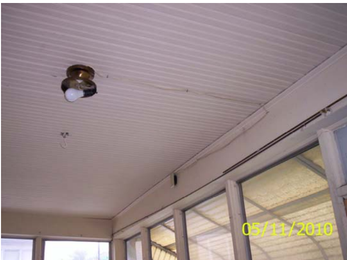
Unapproved electrical wiring on front porch
