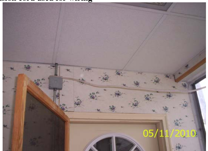
Unapproved electrical wiring on rear porch
