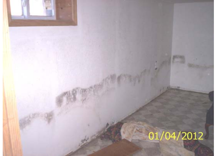
Water damaged wall, mold
