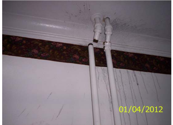
Blown out hot water heating line
