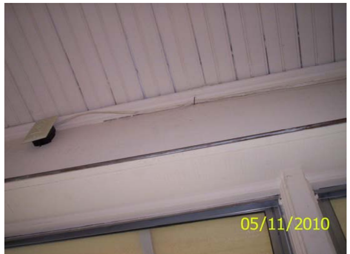
Unapproved electrical wiring on front porch
