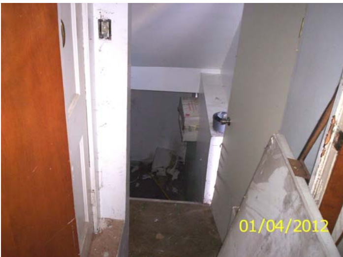
Missing cover plate, exposed wiring, damaged door frame
