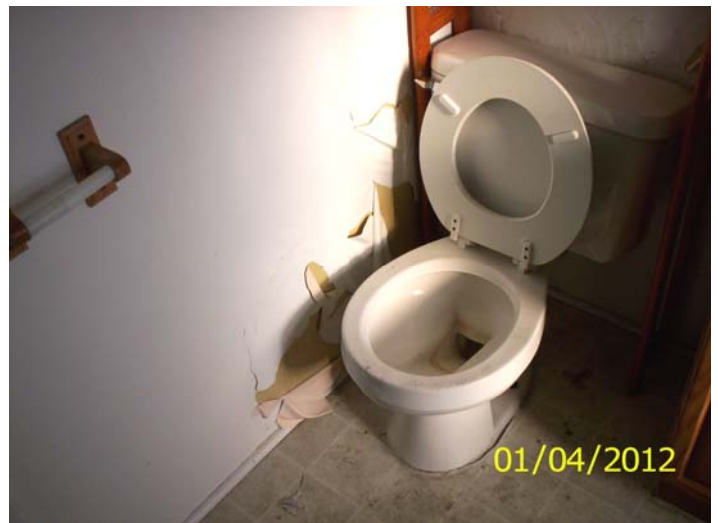
Chipped/peeling paint, dry water trap, open floor covering
