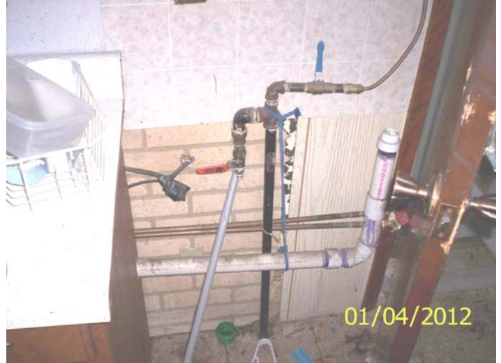
Improper electrical splice, open plumbing
