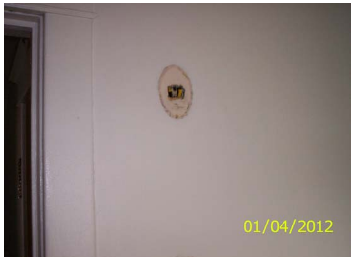
Missing cover plate, exposed wiring
