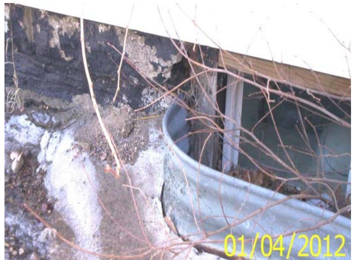
Close view of open foundation, shifted foundation block and missing mortar joint, debris pile
