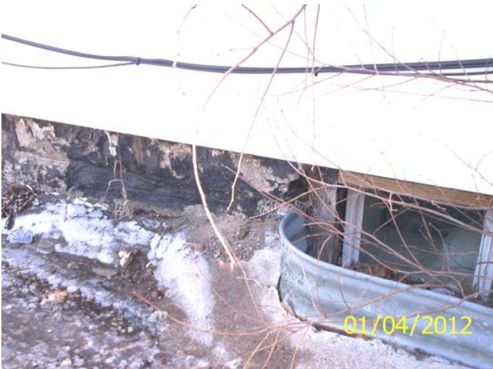
Open foundation wall, shifted block
