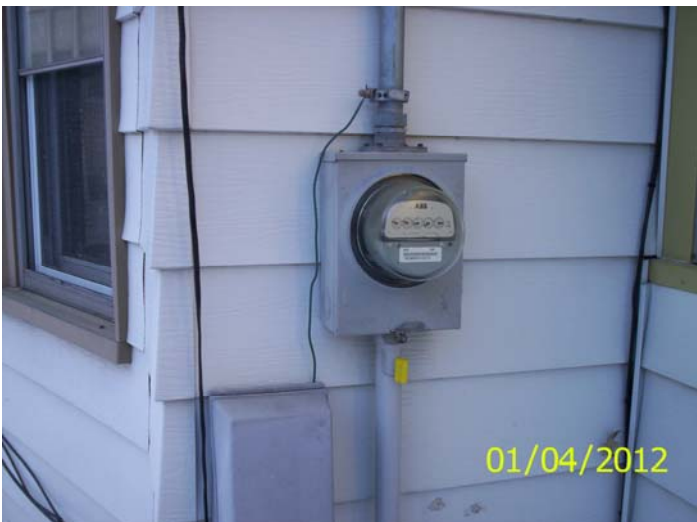
Electric service yellow tagged off
