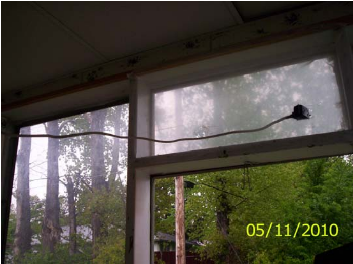
Unapproved electrical wiring on rear porch
