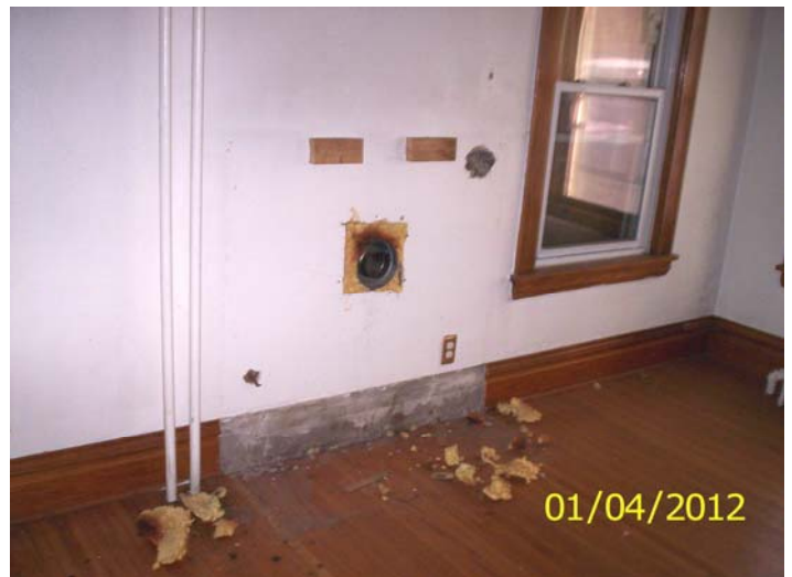
Missing floor board, missing wall mounted heater, open Wall, cut gas line for heater
