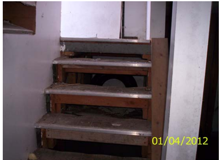
Missing hand rail for basement steps
