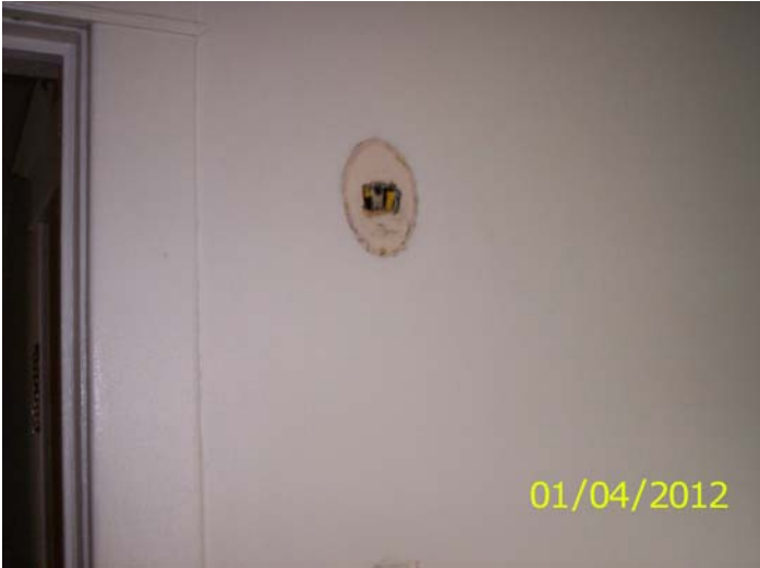
Missing fixture, open electric, exposed wiring
