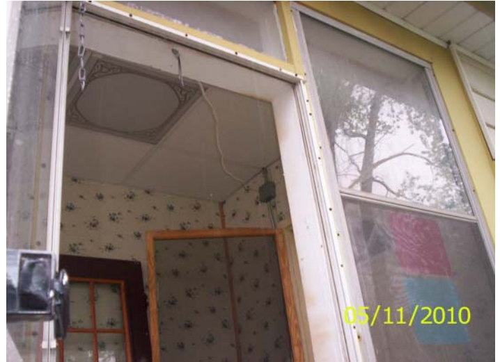
Unapproved electrical wiring on rear porch
