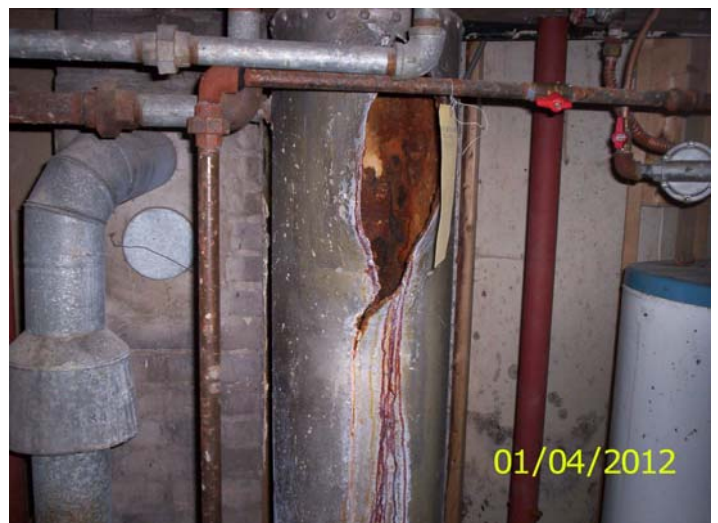
Burst expansion tank for the hot water heating system
