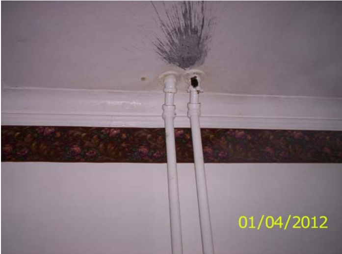
Blown out hot water heating line
