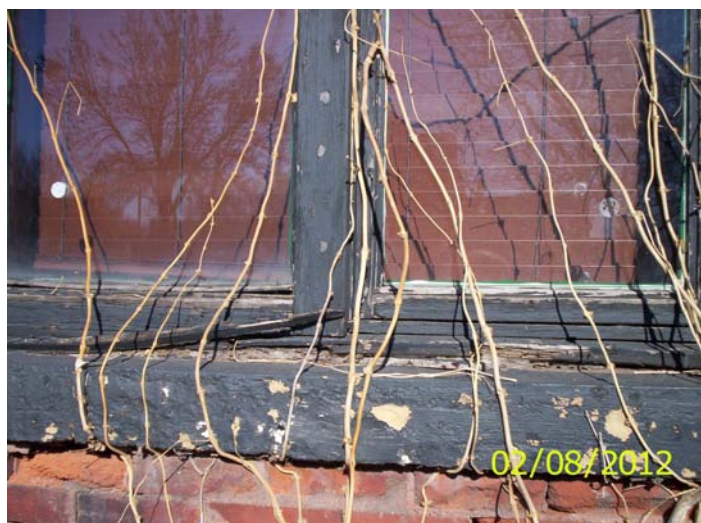
Deteriorated window frame, open wall
