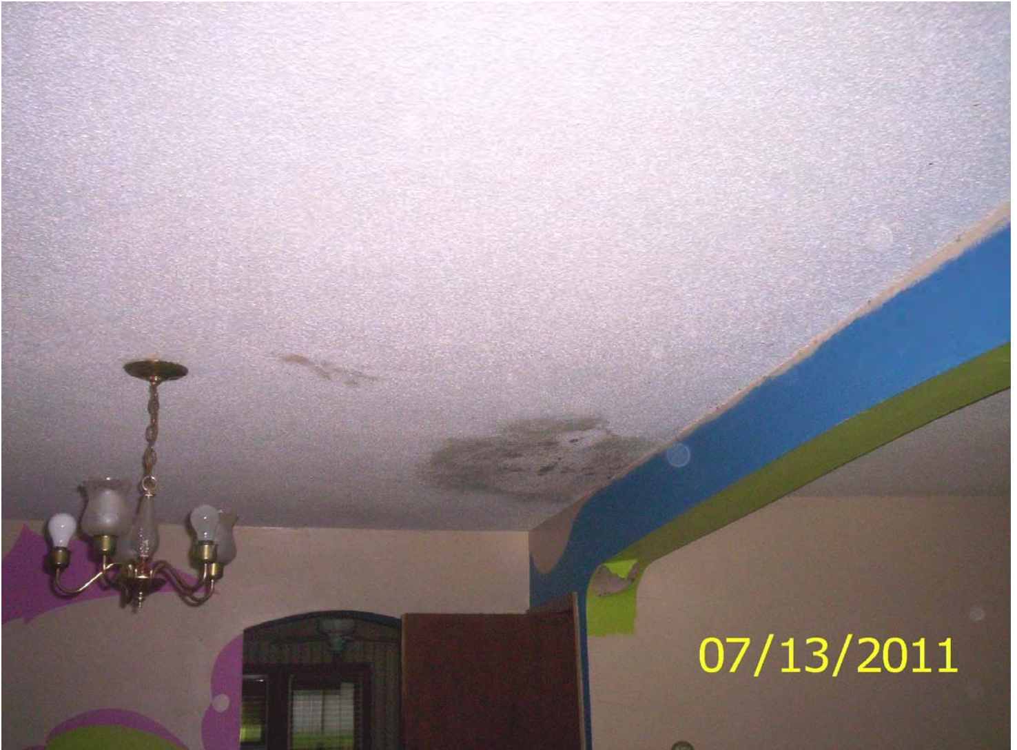
Water damaged ceiling, peeling paint, possibly mold
