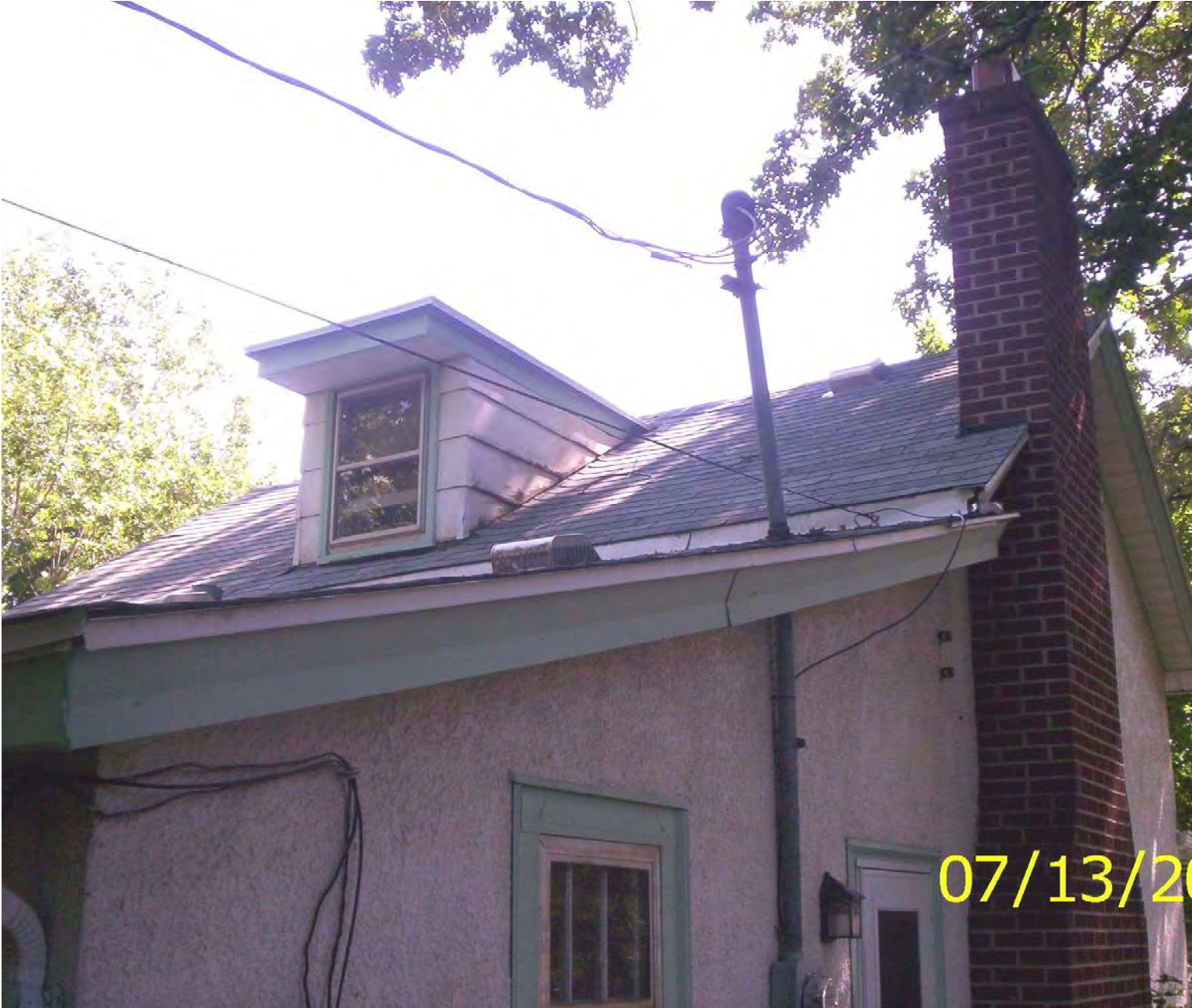
South and west face of the west side dormer, missing flashing, water damaged siding
