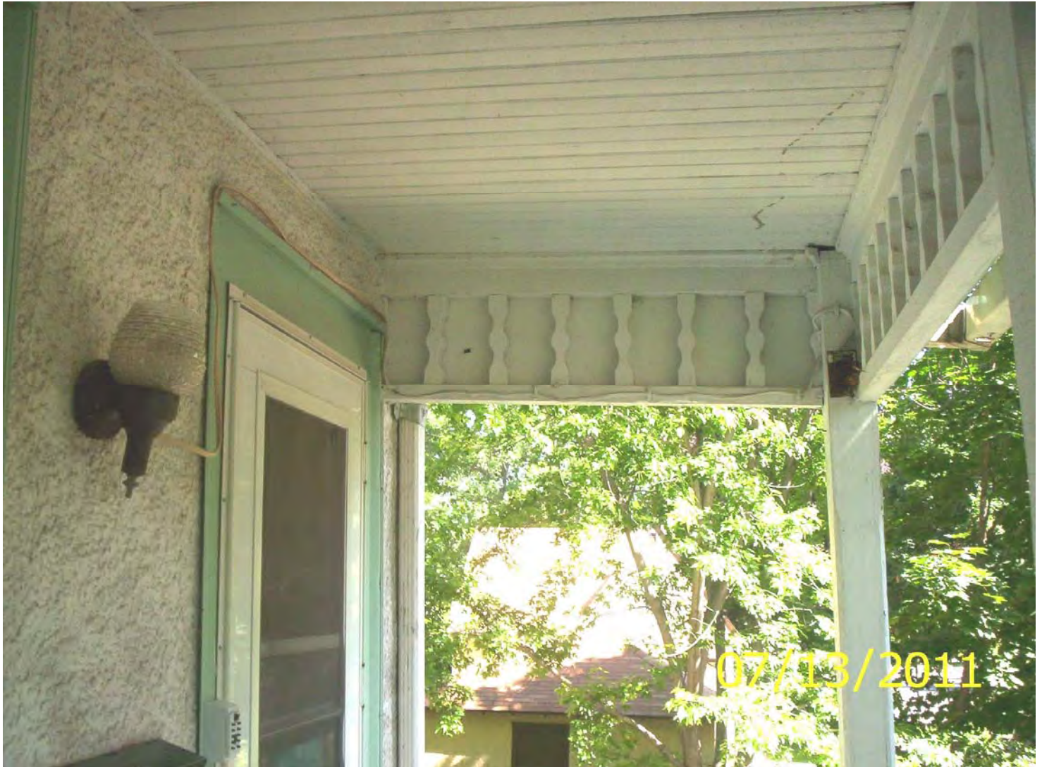
Unapproved exterior electrical wiring
