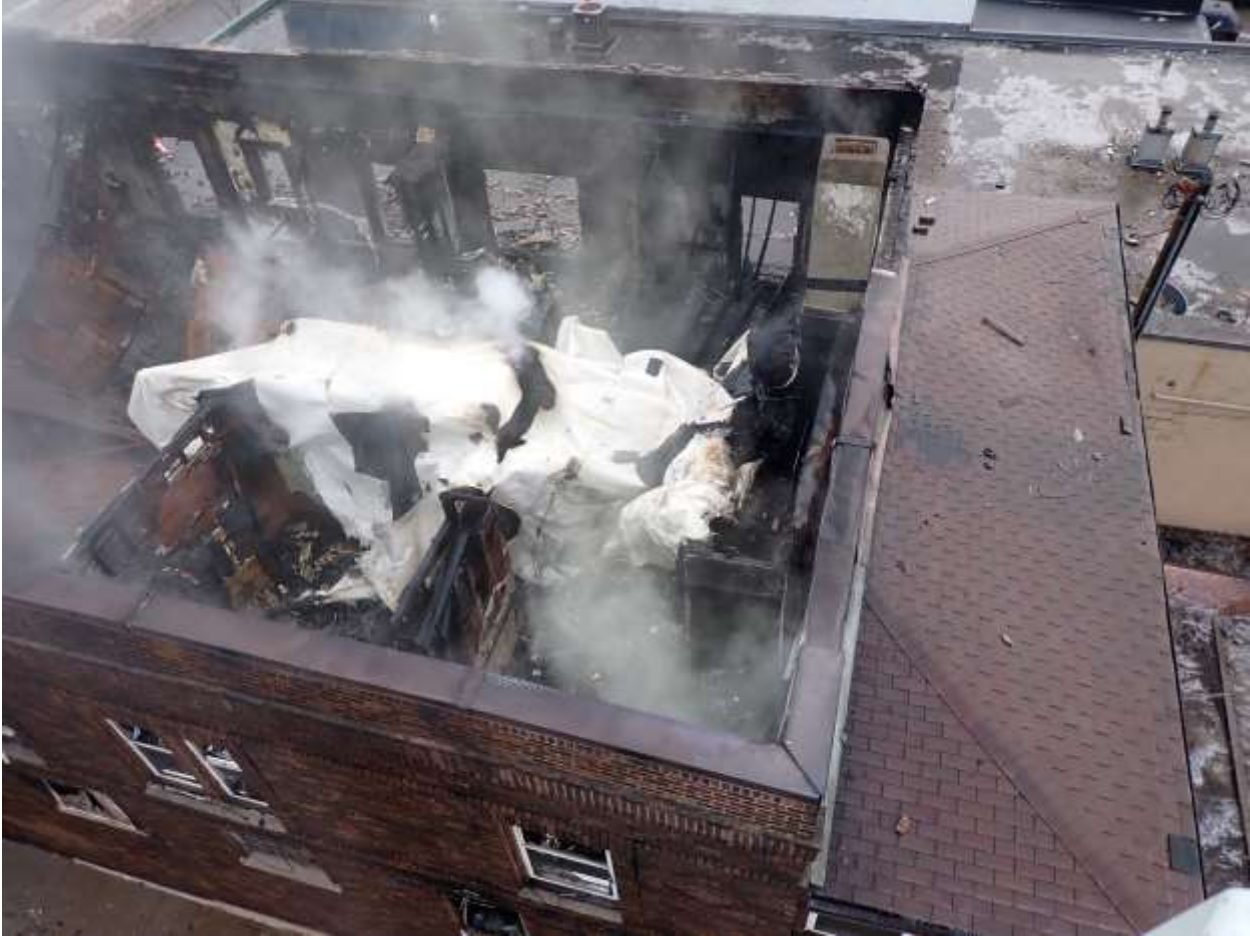
916-918 University Ave W.Fire Photos 1-10-24
