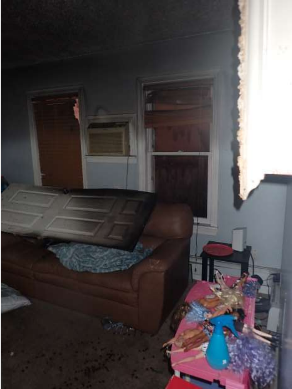
1213 Woodbridge St.Fire Photos 12-1-21
