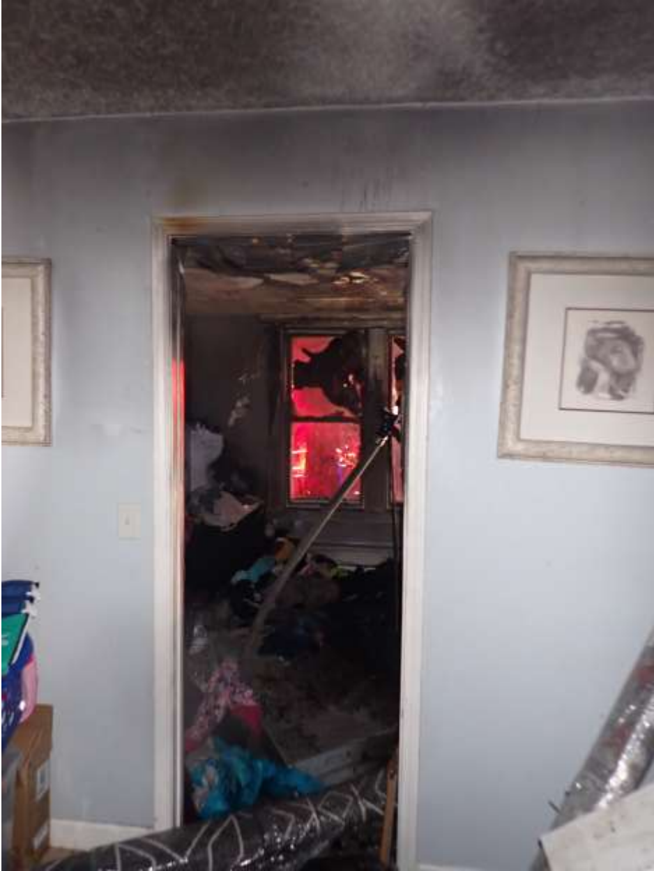
1213 Woodbridge St.Fire Photos 12-1-21
