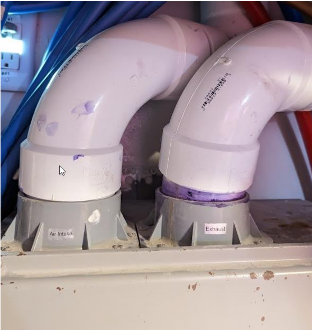
Water Heater Mounted to wall
