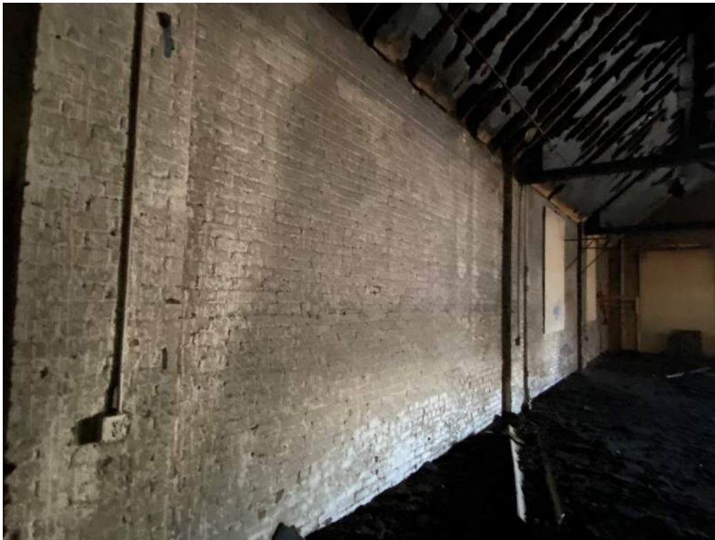
PHOTO #4: View of North wall closest to fire location
