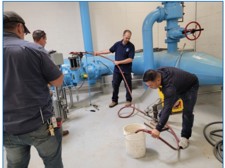
James Lee, maintenance worker, hand pumps to open the discharge valve at the Beebe Road pump station while Jon Hendrickson, Dick Keeney and Jon Falardeaux provide support.
