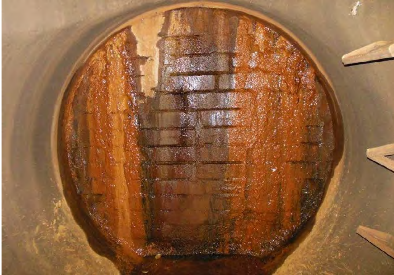
Iron Bacteria on Bulkhead
