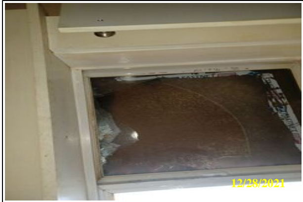
Date Serviced: 12/28/2021 Room: No Room Category: Windows
