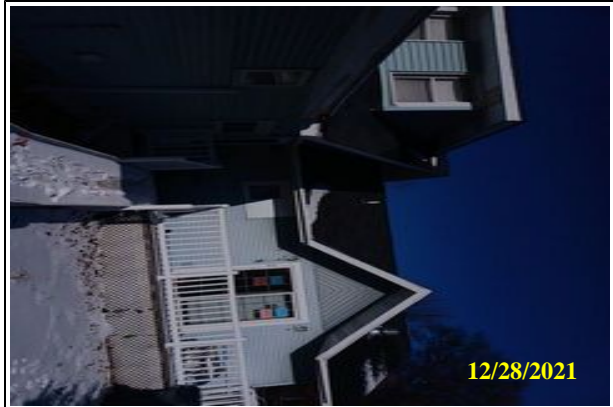
Date Serviced: 12/28/2021 Room: No Room Category: Siding
