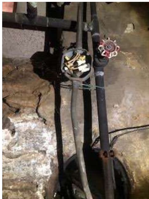
42: Electrical box missing cover
