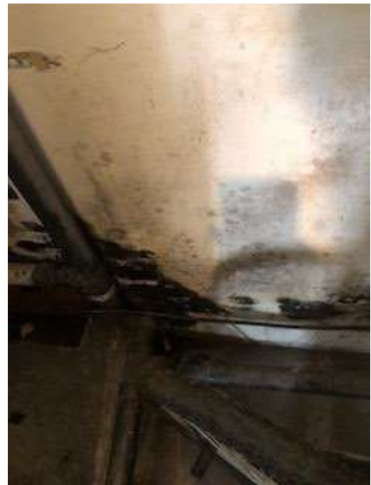
20: Mold at laundry room walls
