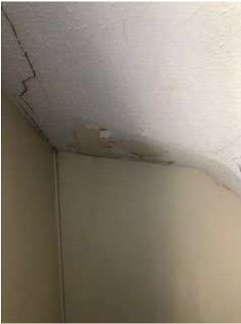
21: Ceiling flaking and cracking in hallway
