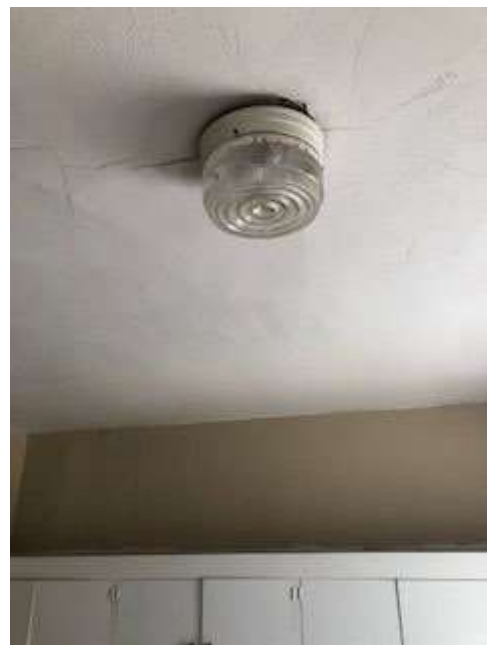
28: Cracking near light fixture in tenant unit
