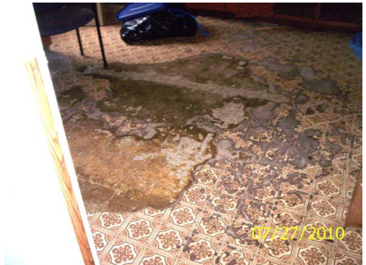
Deteriorated kitchen floor
