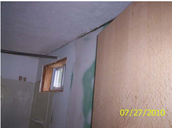
Unfinished remodel of bathroom, no permits
