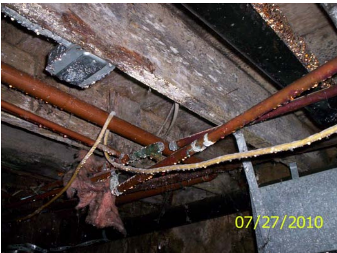
Improper electrical wiring, no permit for work
