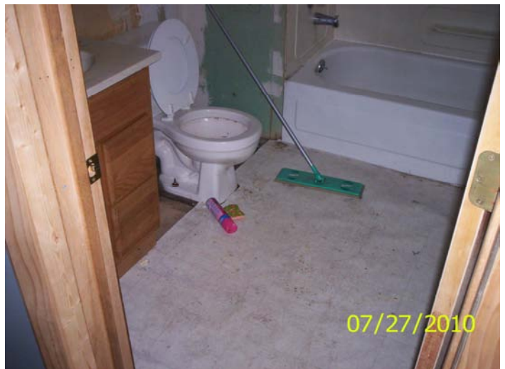
Unfinished bathroom floor, no permit
