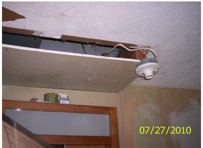
Improper electrical wiring in bathroom, no permit
