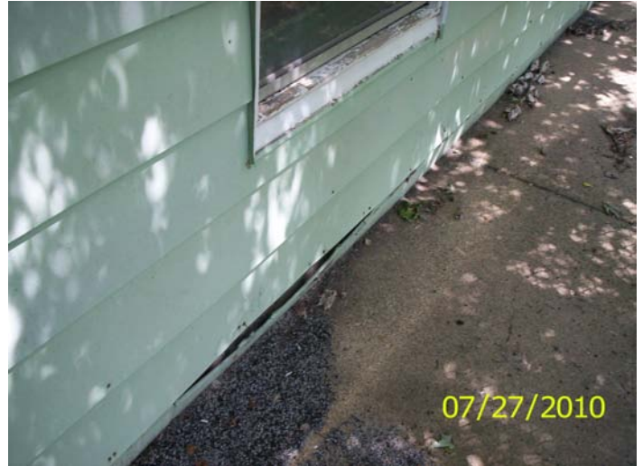
Siding/trim coming off of wall
