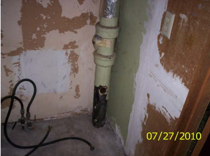
Open main plumbing stack, improper repair
