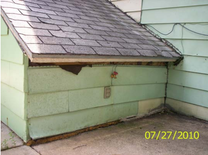
Missing, deteriorated siding
