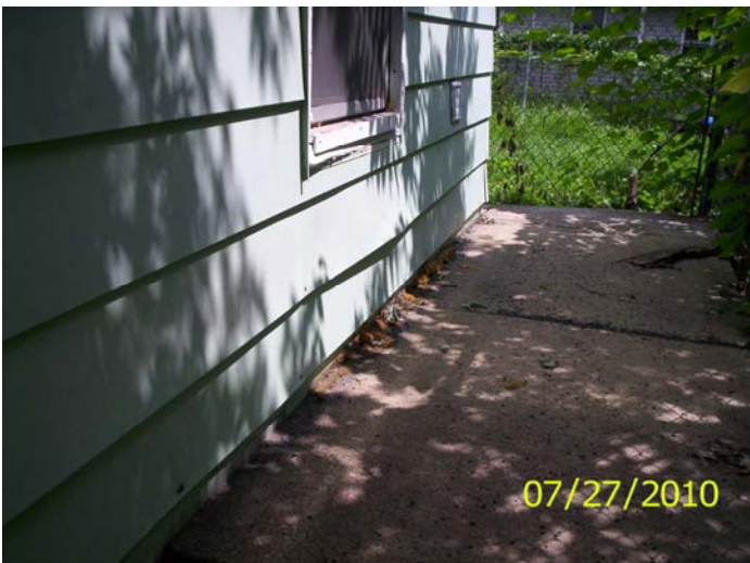
Siding coming off of wall
