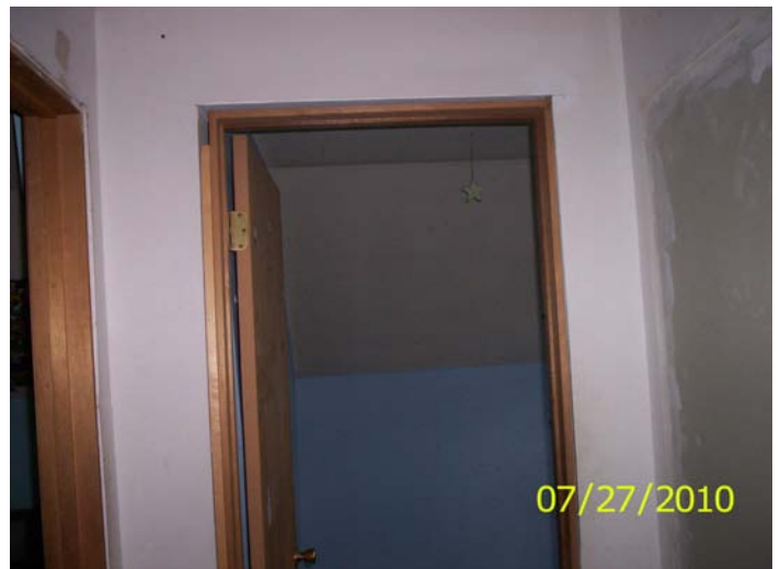
Unfinished remodeling, no permits
