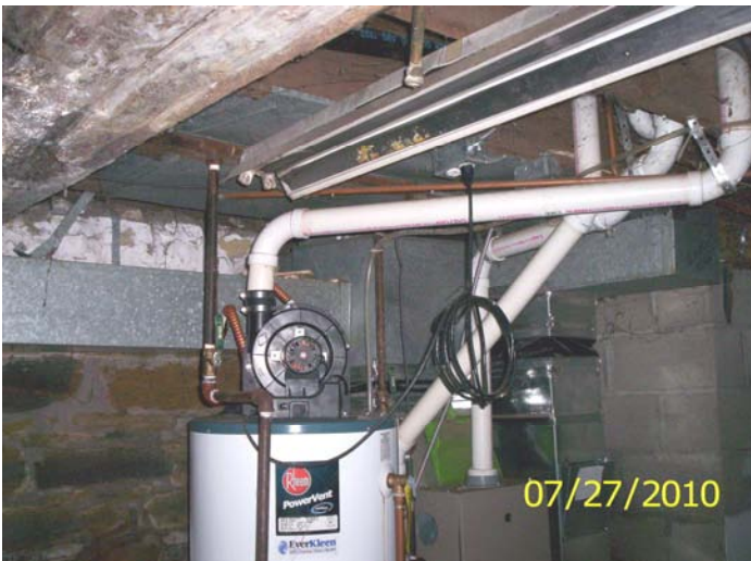
Improper installation of water heater, no permit
