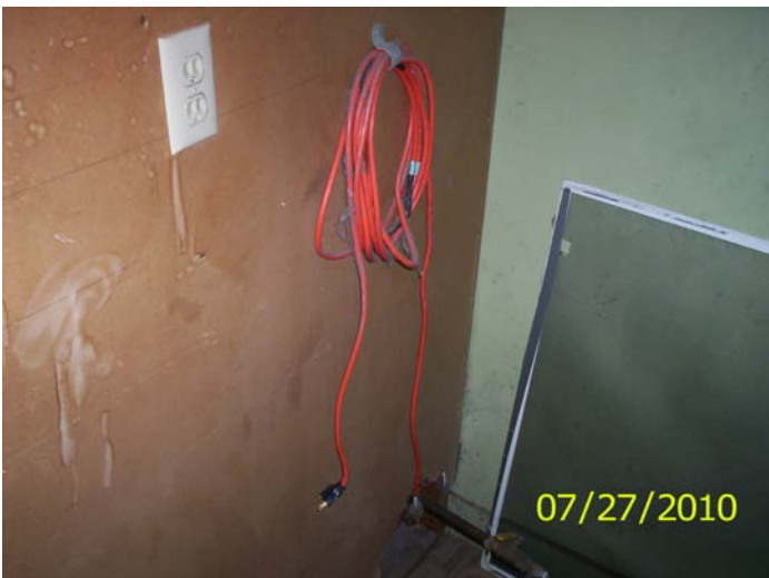
Extension cord wiring
