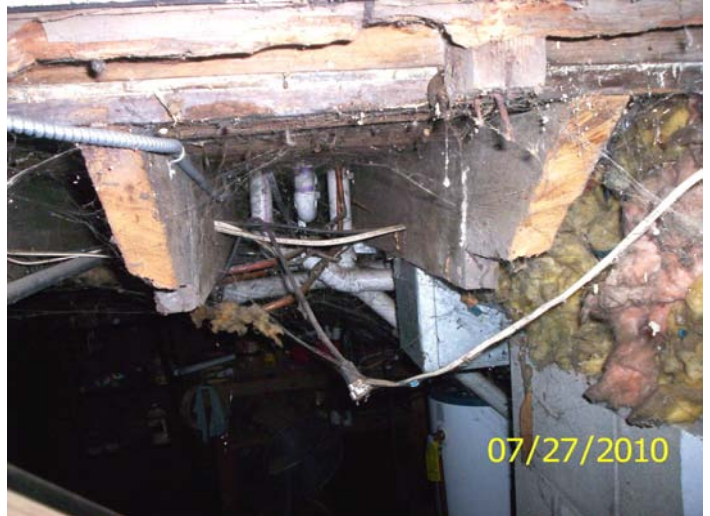
Improperly terminated floor joists, extension cord wiring
