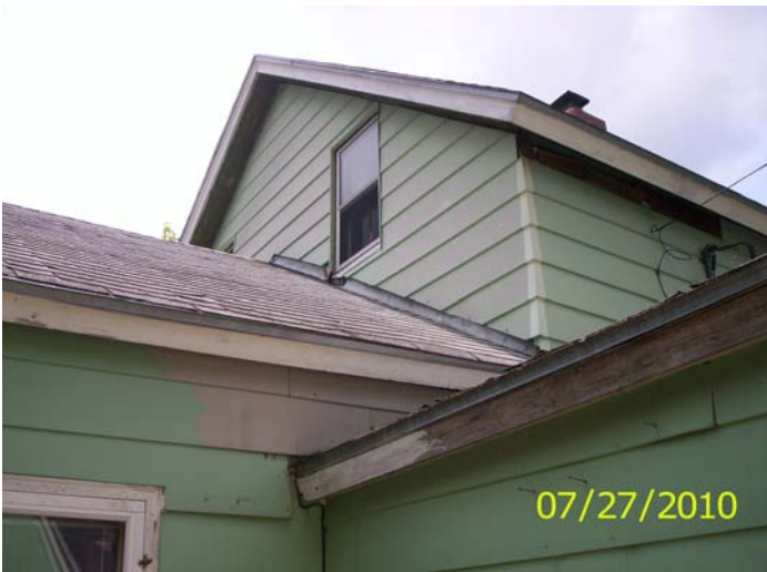
Unfinished siding installation, exposed wood surfaces, Improper flashing
