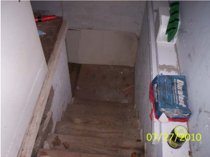
Stairs to basement, no hand rail
