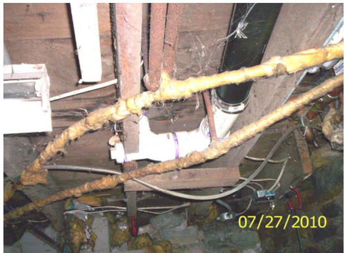
New plumbing and electrical installations, no permit
