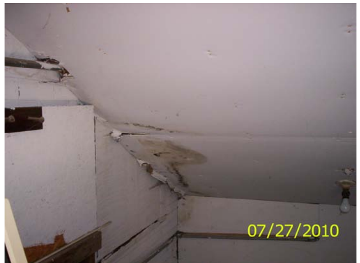
Water damage to ceiling in stair way to basement
