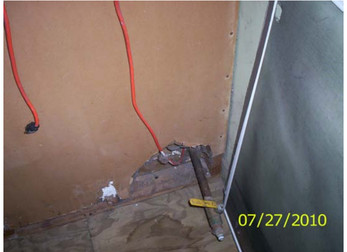
Extension cord wiring going into wall
