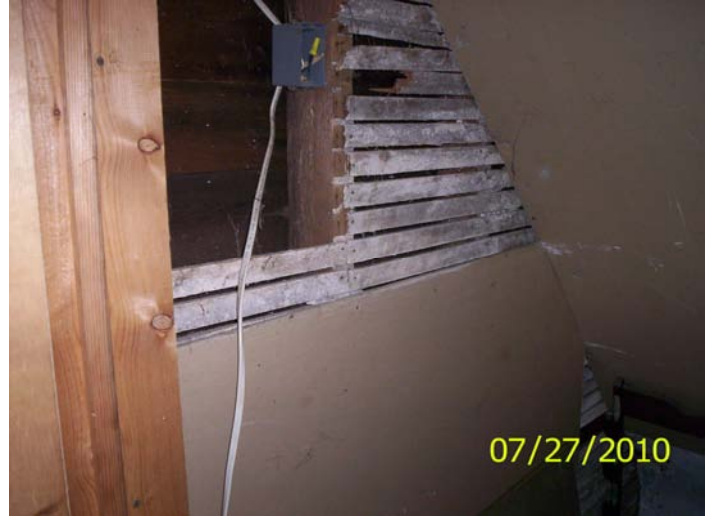
Open wall, improper electrical installation, no permits
