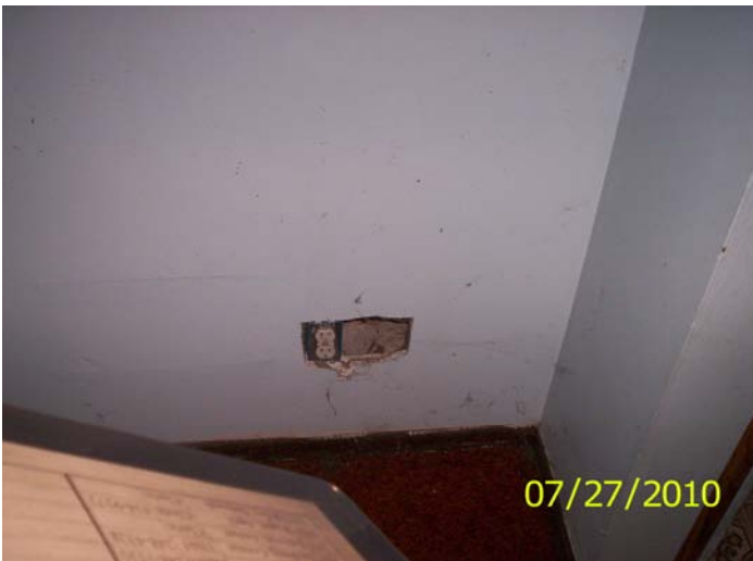
Hole in wall for electrical outlet installation, no permit
