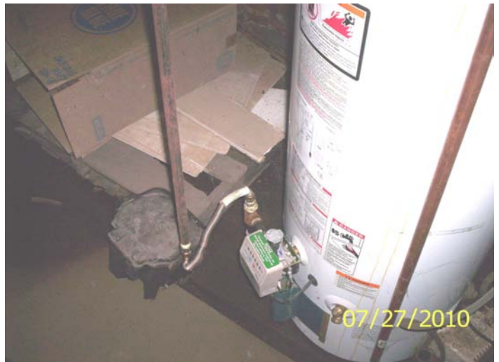
Flexibile gas line connection crimped at both ends, t/p valve spill tube too close to floor, no permit for work
