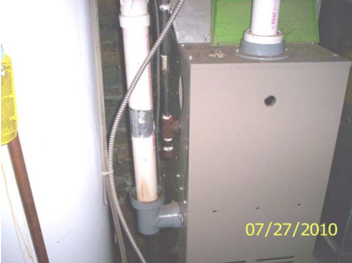
Improper pipe union
