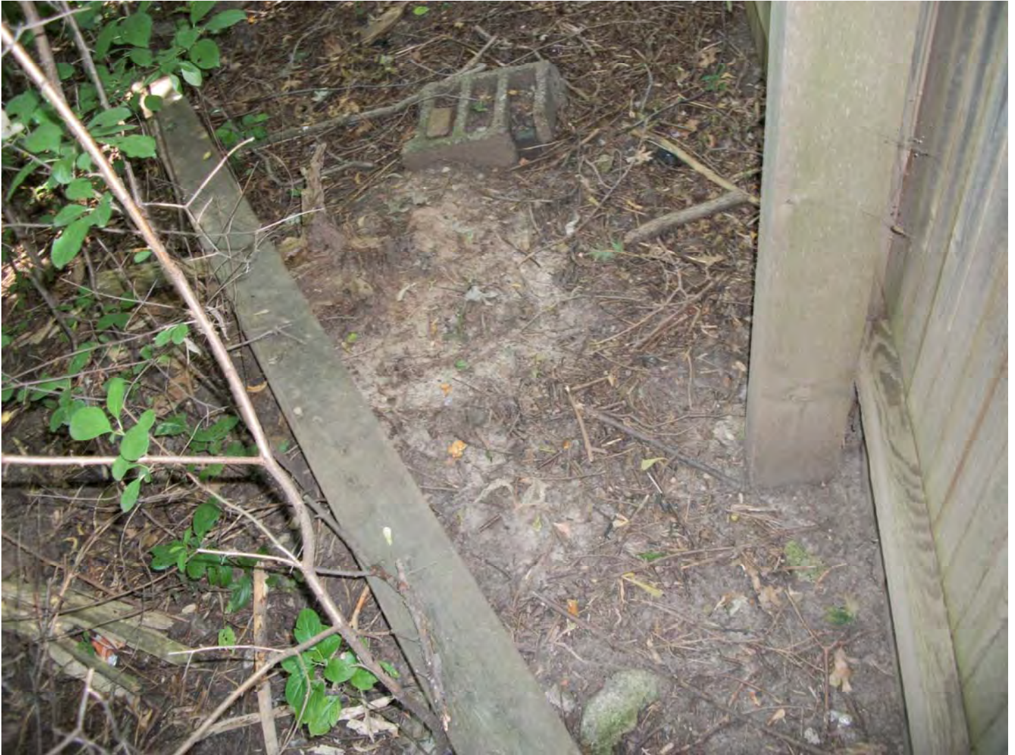
21 East section, broken support
