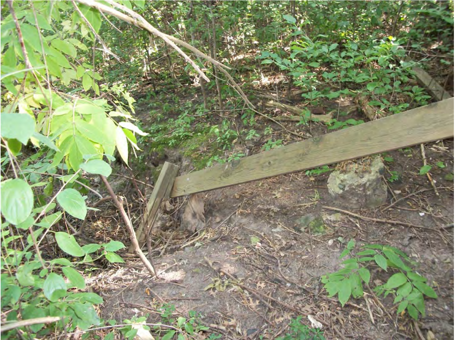
20 East section, damaged support
