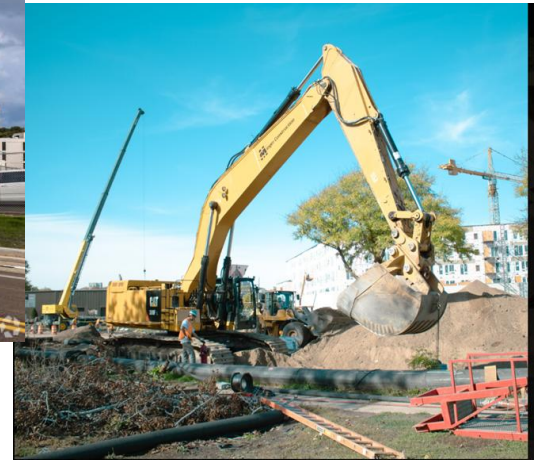
Water Street Sanitary Sewer Lift Station
