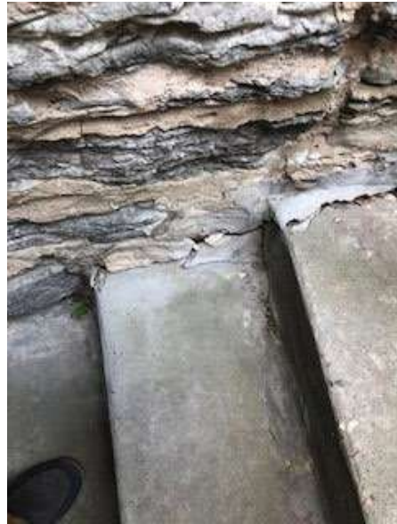
14: Mortar gaps at concrete steps to Unit 5
