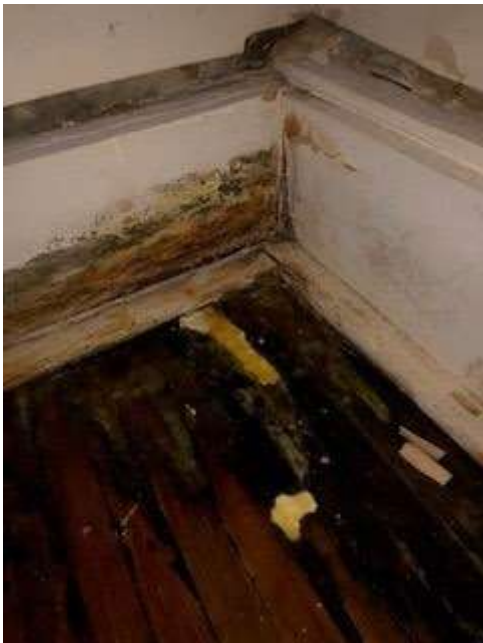
23: Mold/rot at baseboards and flooring
