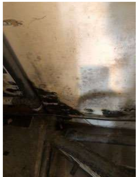
20: Mold at laundry room walls
