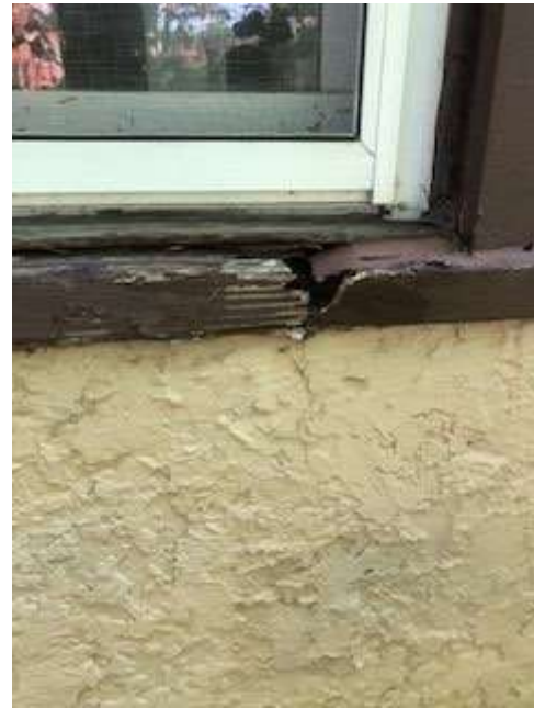
4: Rotting/peeling exterior trim and cavity
