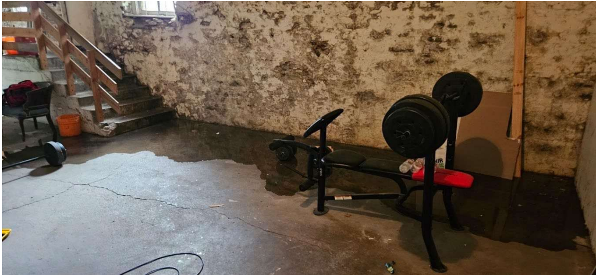
12: Water infiltration and flooding in entry/storage to Unit 5 due to deteriorating foundation (photograph taken by Mr. Cornell on June 16, 2025)
