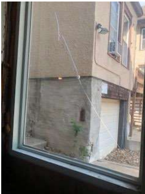
36: Cracked window in laundry room
