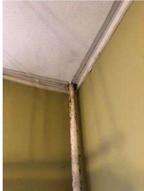
26: Mold/rust on exposed pipe
