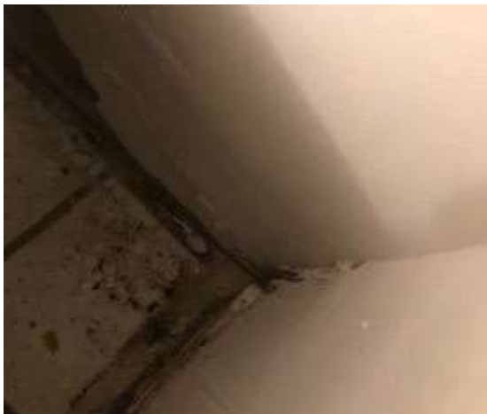
30: Damaged flooring in tenant unit
