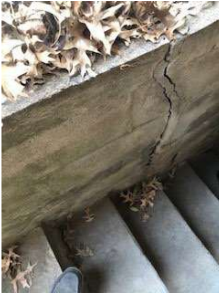
13: Cracks at concrete steps to Unit 5
