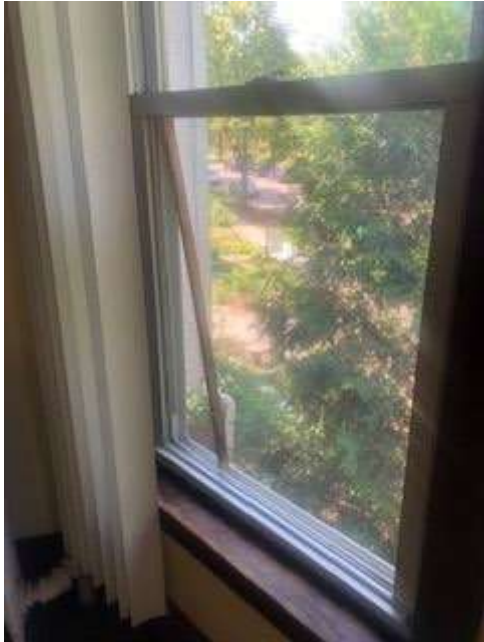
34: Tenant window held up by wooden post
