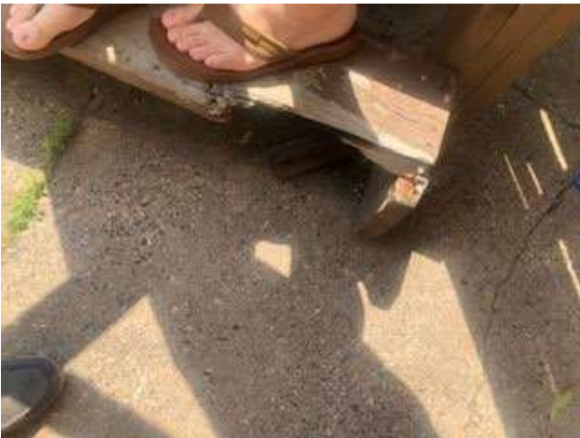
6: Broken step at rear stairs to unit entry
