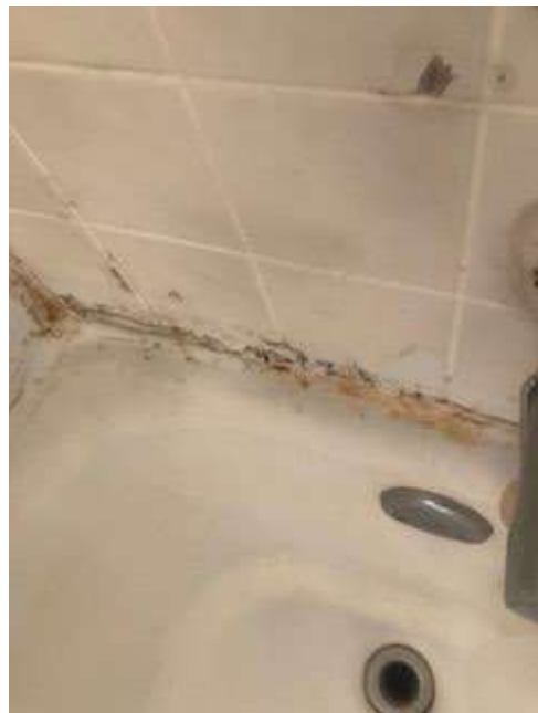
24: Mold and deterioration in unit shower
