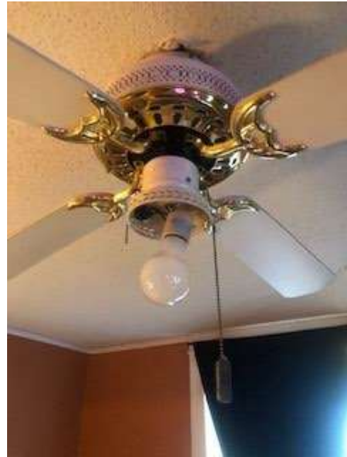
44: Wobbly fan in tenant unit w/o cover
