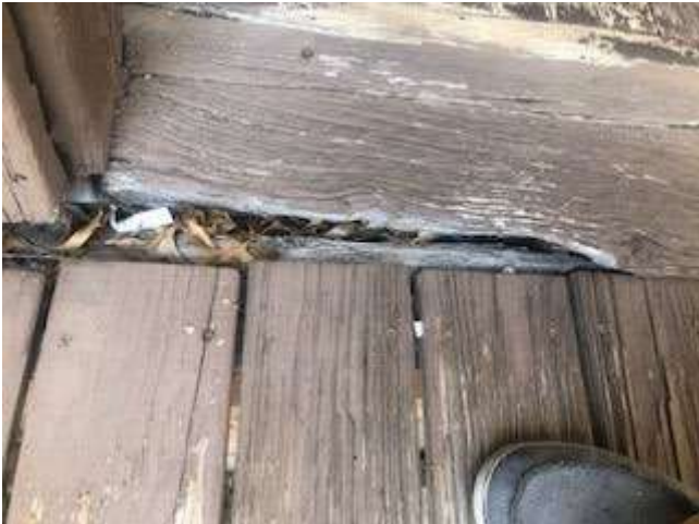
7: Cracked wood at top step for rear stairs to unit entry
