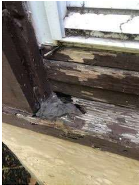
2: Rotting/peeling exterior trim and cavity
