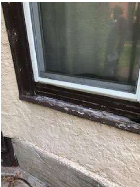
3: Rotting/peeling exterior trim
