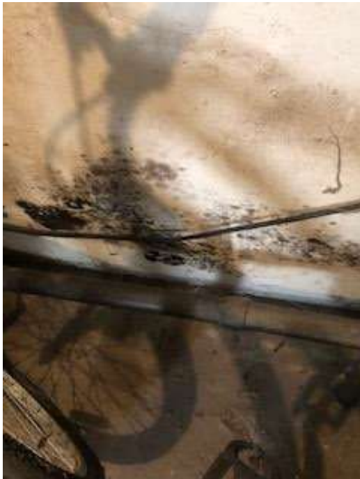
19: Mold at laundry room walls
