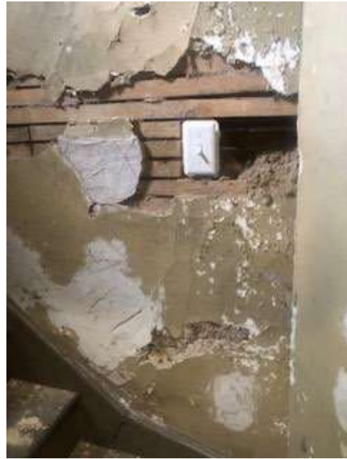
22: Wall deterioration at stairway
