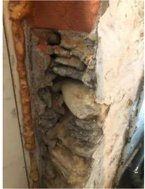
11: Settling foundation with holes
