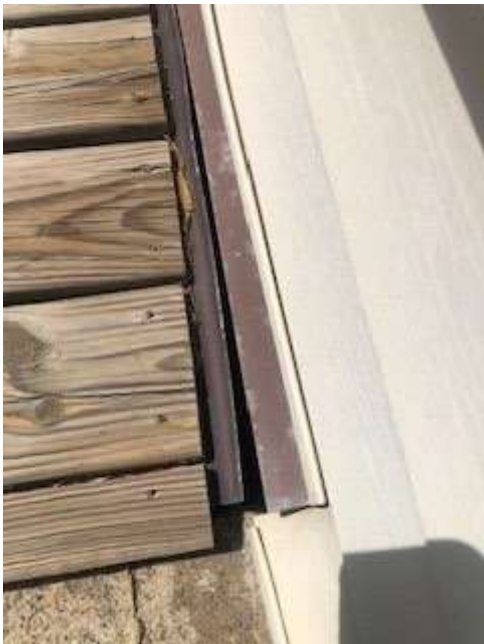
5: Wooden balcony separating from siding
