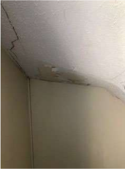
21: Ceiling flaking and cracking in hallway
