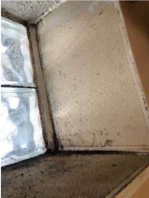
25: Mold at glass block window in unit shower
