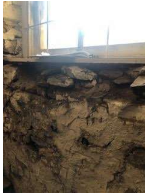
9: Deteriorating foundation at basement window
