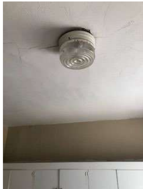
28: Cracking near light fixture in tenant unit
