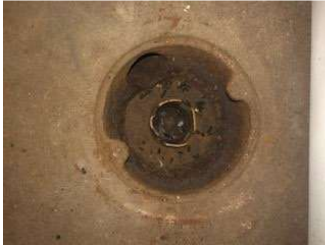
39: Laundry room floor drain missing clean-out plug, with rodent feces present
