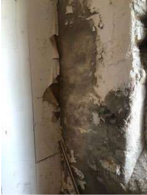
10: Flaking paint and worn foundation
