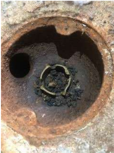
40: Unit 5 storage area floor drain missing clean-out plug
