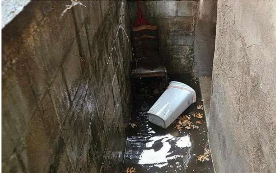
16: Flooding resulting from gaps and cracks at concrete outside entry to Unit 5 (photograph taken by Mr. Cornell on June 16, 2025)
