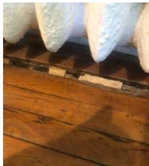
31: Crack in floor under radiator in tenant unit
