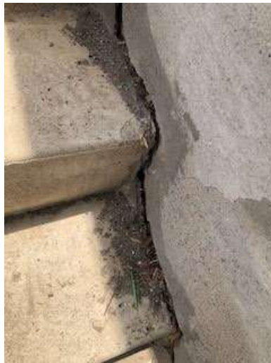
15: Mortar gaps at concrete steps to Unit 5
