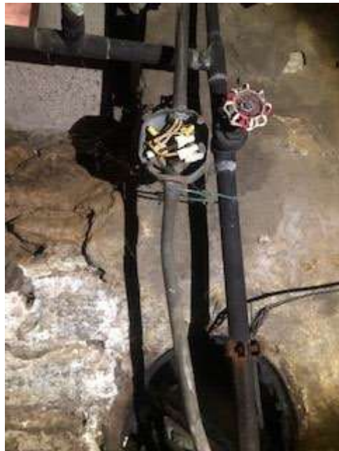
42: Electrical box missing cover
