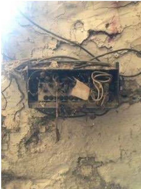
41: Electrical box missing cover
