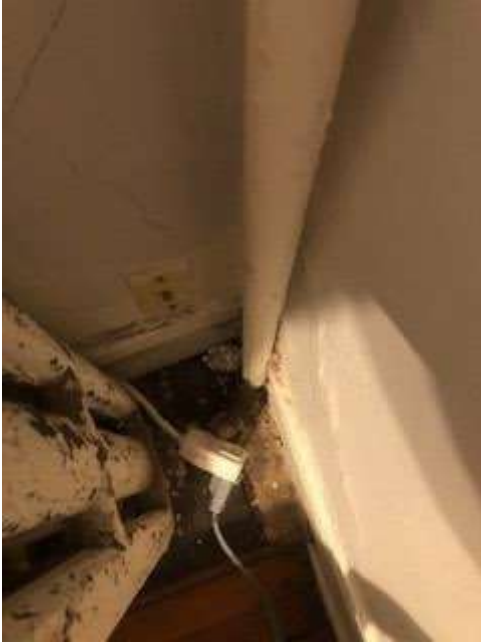
32: Missing flooring in tenant unit
