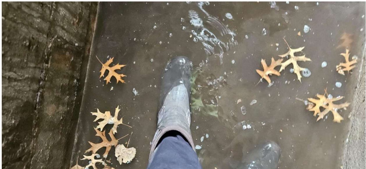
17: Several inches of water from flooding at entry to Unit 5 (photograph taken by Mr. Cornell on June 16, 2025)
