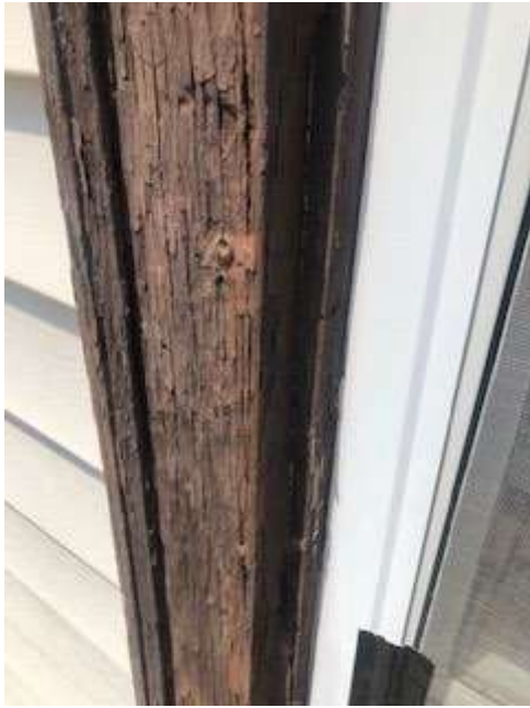
1: Rotting/peeling exterior trim
