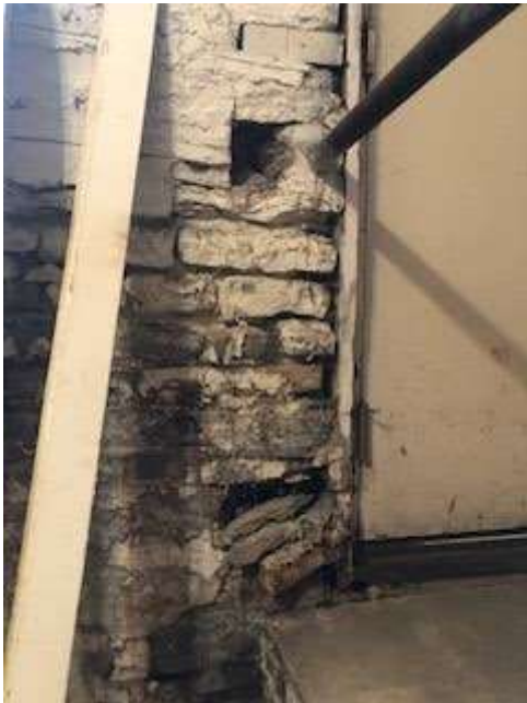
8: Settling and holes in foundation
