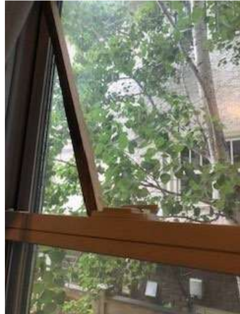
35: Tenant window held up by wooden post
