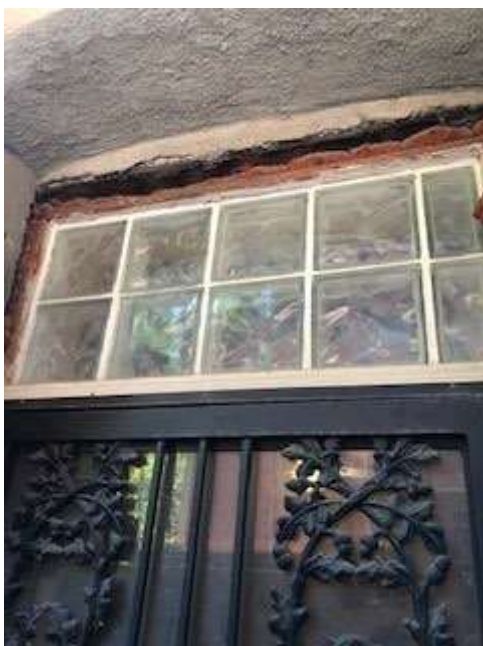
18: Gaps at glass above exterior door to Unit 5
