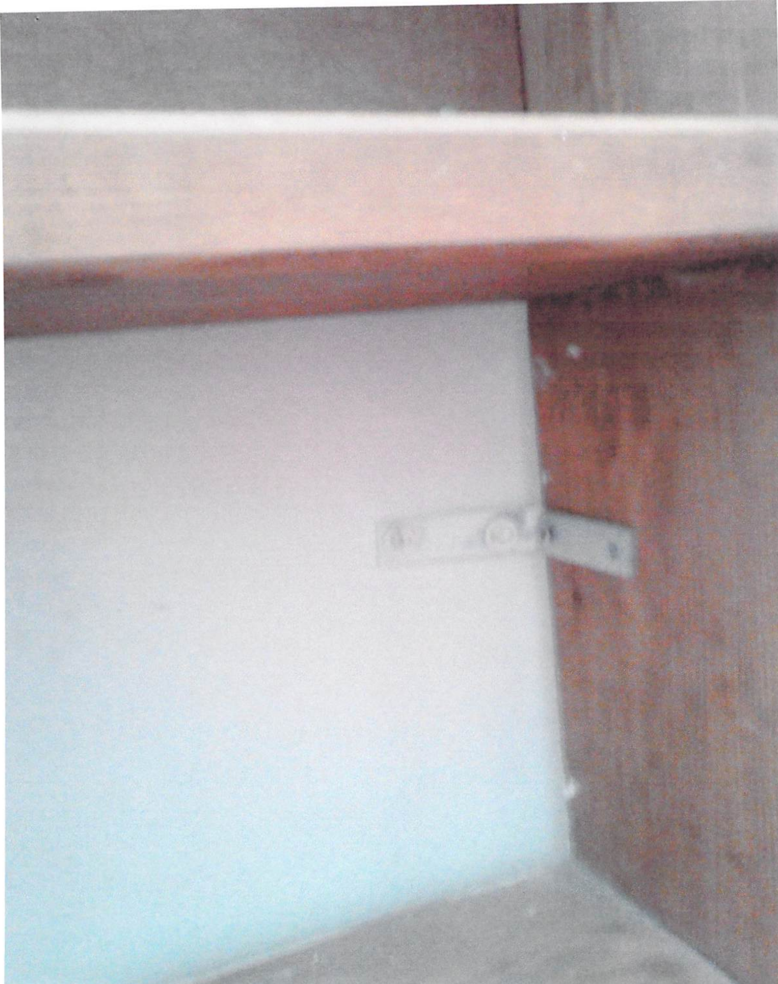
Unit 1 missing Screw
