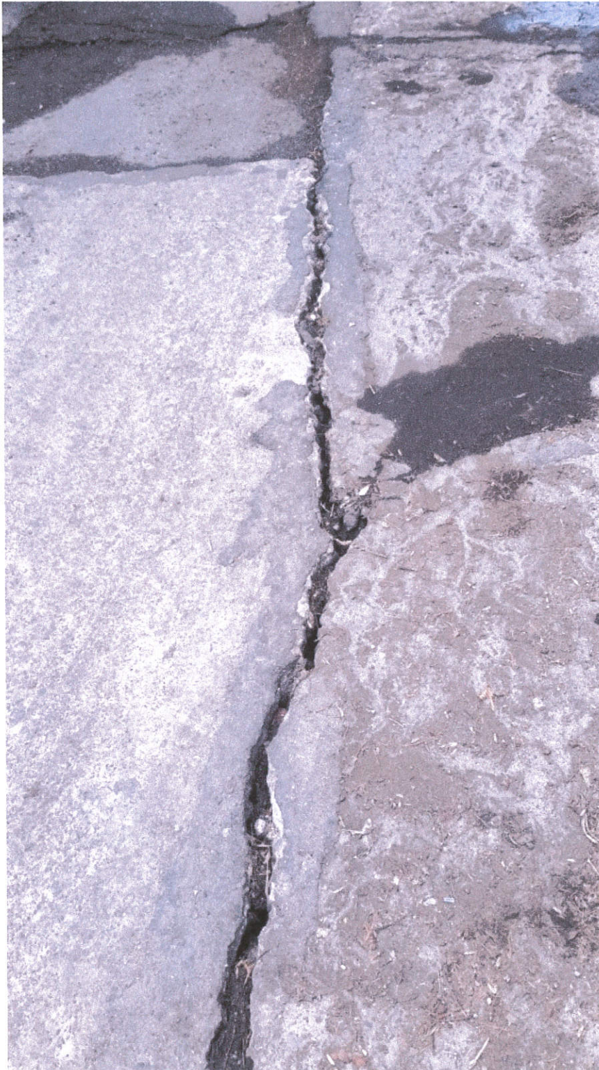
Detail picture of public alley showing severe cracking dated 4/8/2014
