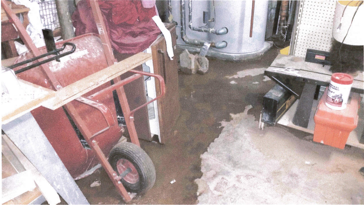
Interior picture of Ashland Apartments basement boiler room dated 1/8/2016. Water on floor is ground water seeping in through basement walls.
