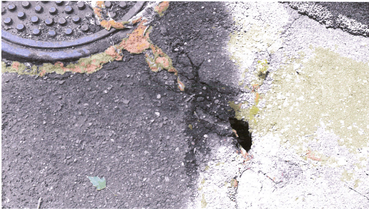
Detail shot of hole by Xcel Energy utility vault dated 7/15/2015
