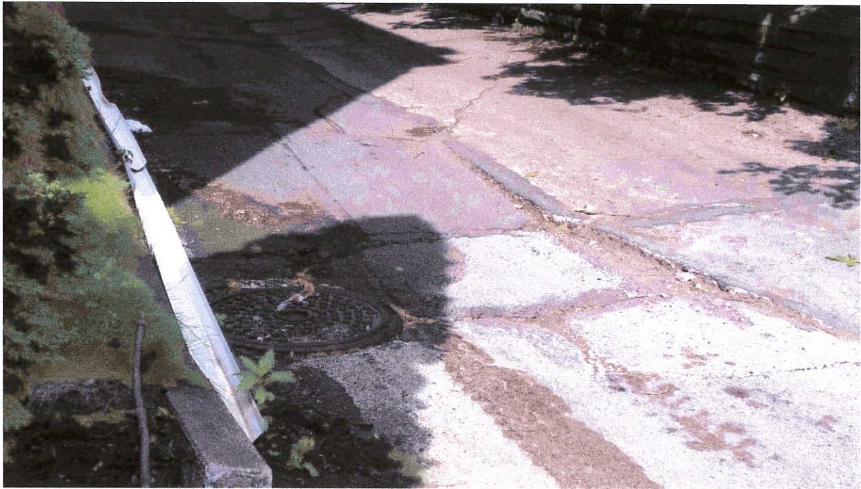
Picture of public alley showing severe cracking and movement of surface pieces dated 7/15/2015
