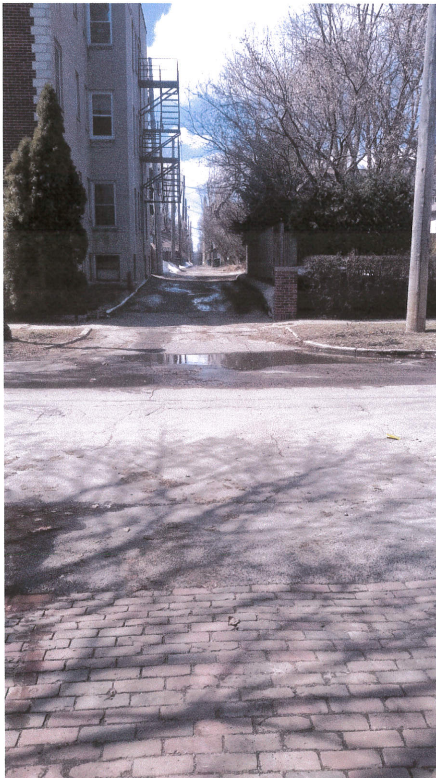
West facing picture of public alley showing ponding of water at street curb cut dated 4/8/2014
