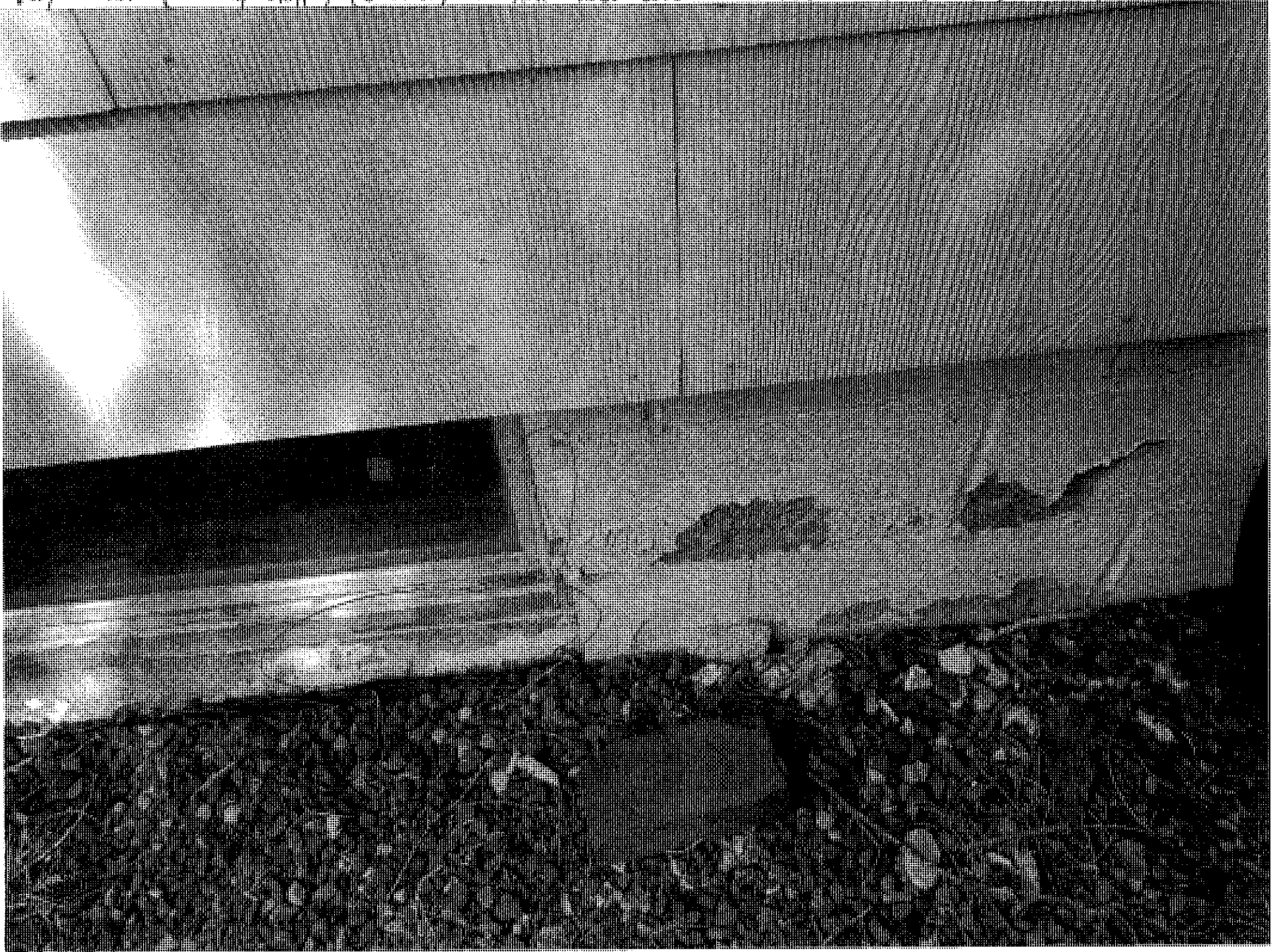
Very minor (41 cm) chipping (cracks) of steel near base of base, circular joint visible
