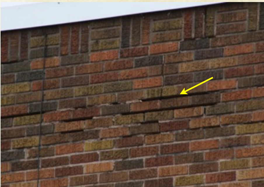
Tuckpointing and brick repairs needed around the entire building.
