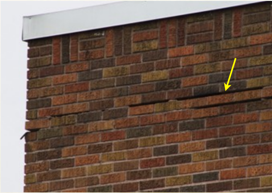
Typical joints needing tuckpointing.
