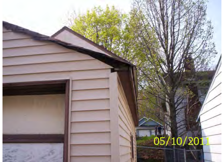
Open siding, water damaged open eave
