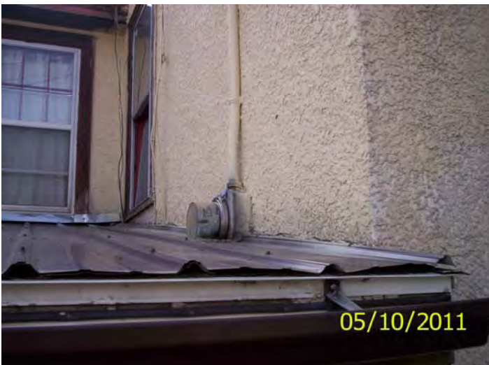
Electric meter buried in roof installation
