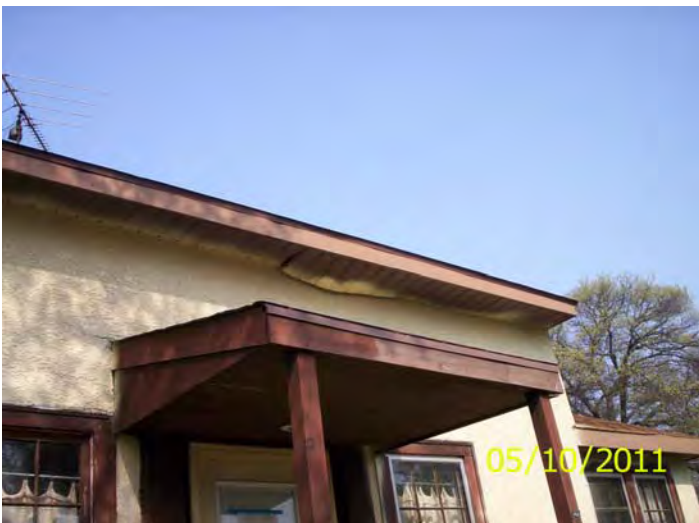
Deteriorated eave covering
