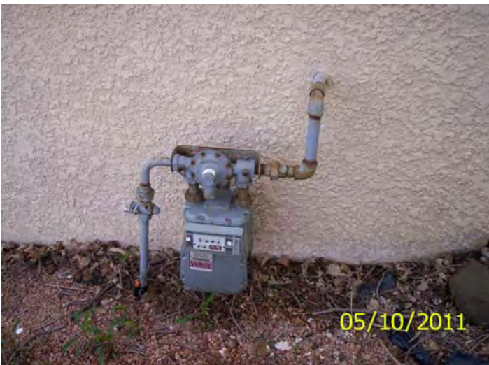
Locked gas meter
