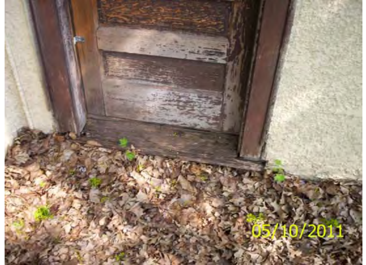
Rot damaged door trim, threshold, framing
