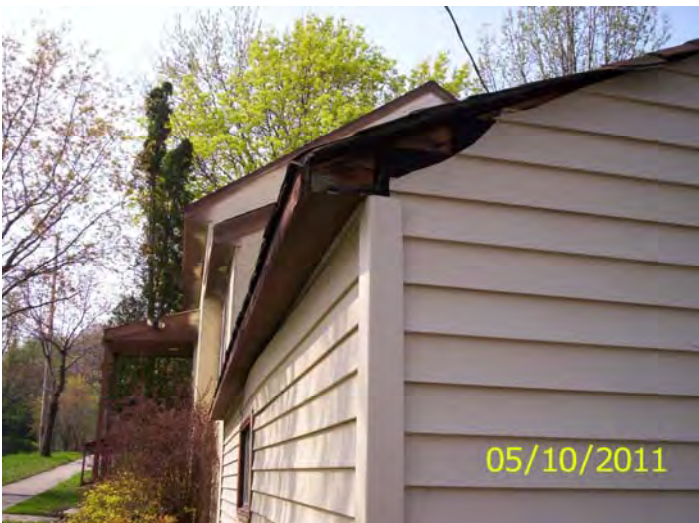
Open siding, deteriorated siding, water damaged open eave
