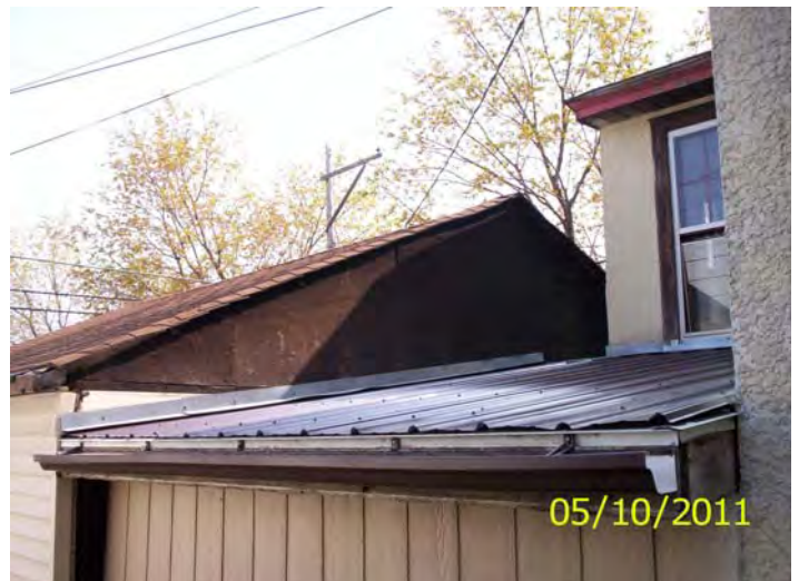
Missing siding, unapproved flashing
