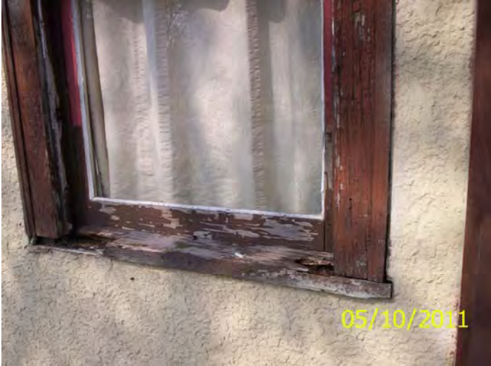
Rot damaged window sash, trim, framing
