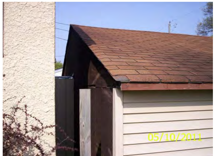
Missing siding, open wall
