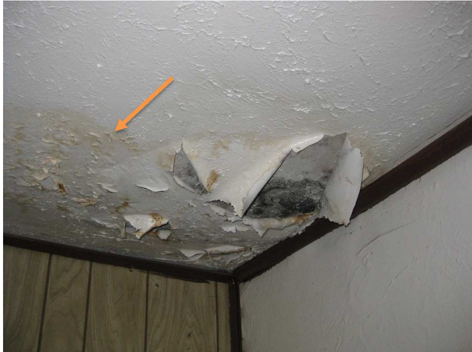
Picture 5 – Water Damage on Second Floor Ceiling
