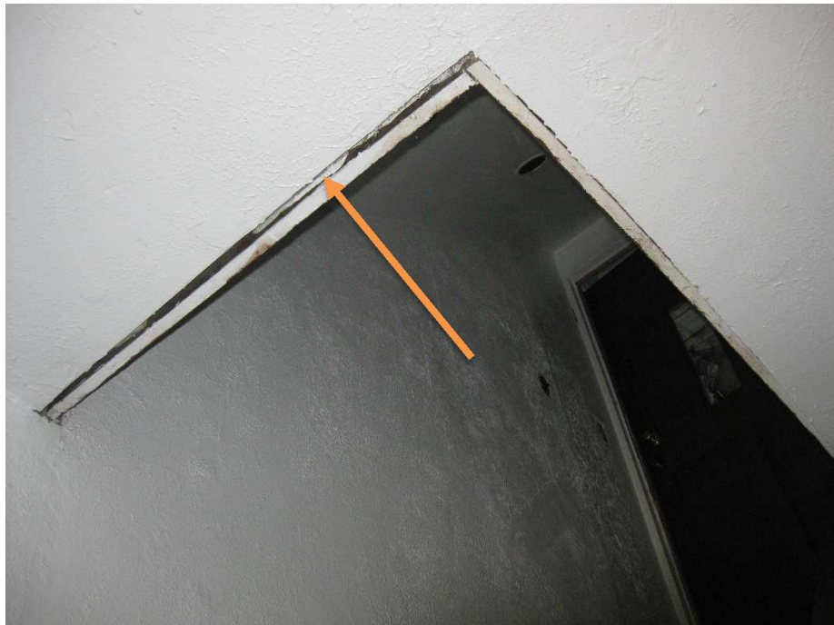
Picture 4 – Gap Due to Sloping
