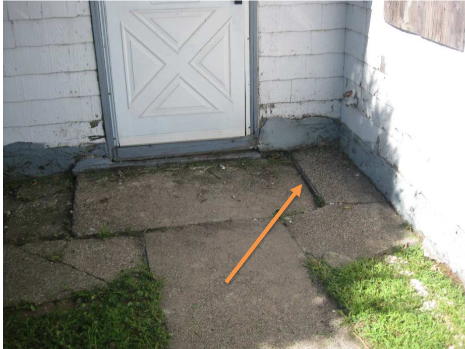
Picture 2 – Front Slab Settlement
