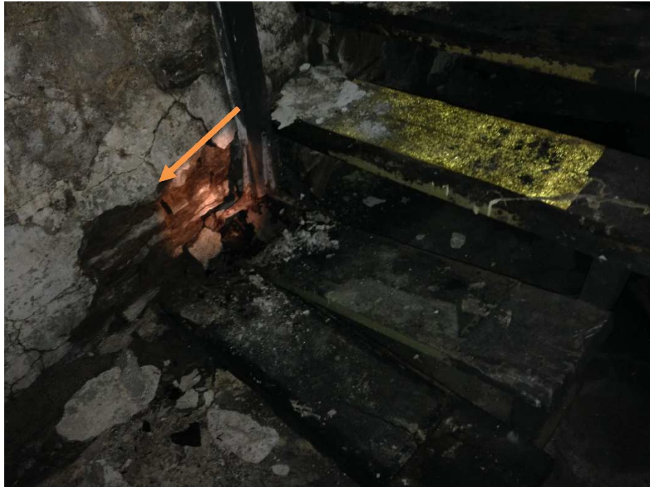
Picture 7 – Crumbling and Cracking of Foundation Walls
