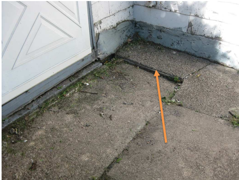
Picture 1 – Front Slab Settlement
