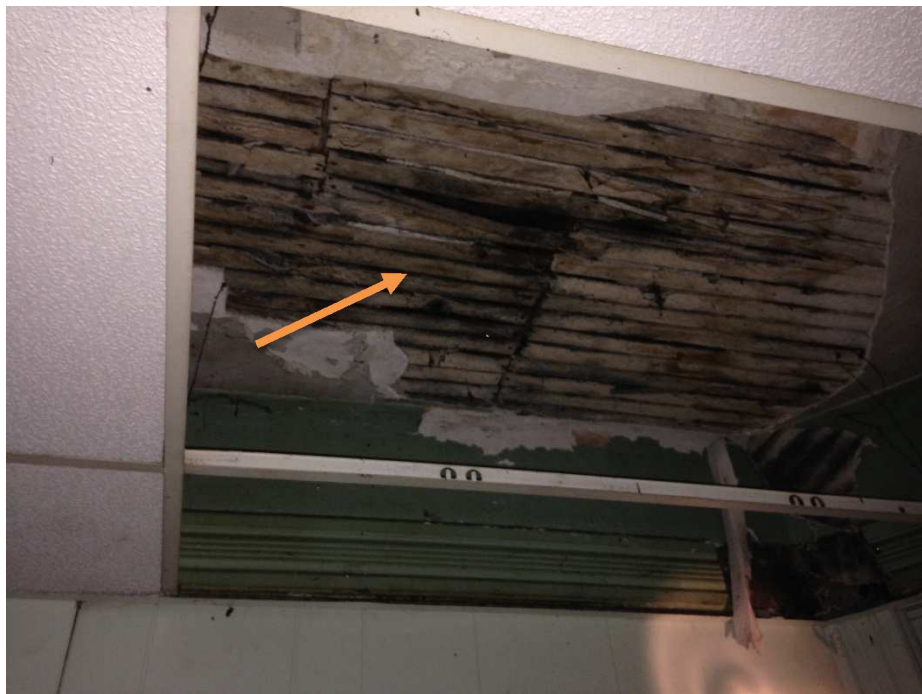
Picture 6 – Deterioration of Ceiling System
