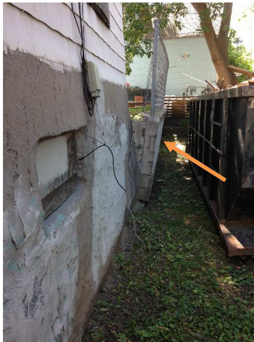
Picture 10 – Retaining Wall Out of Plumb
