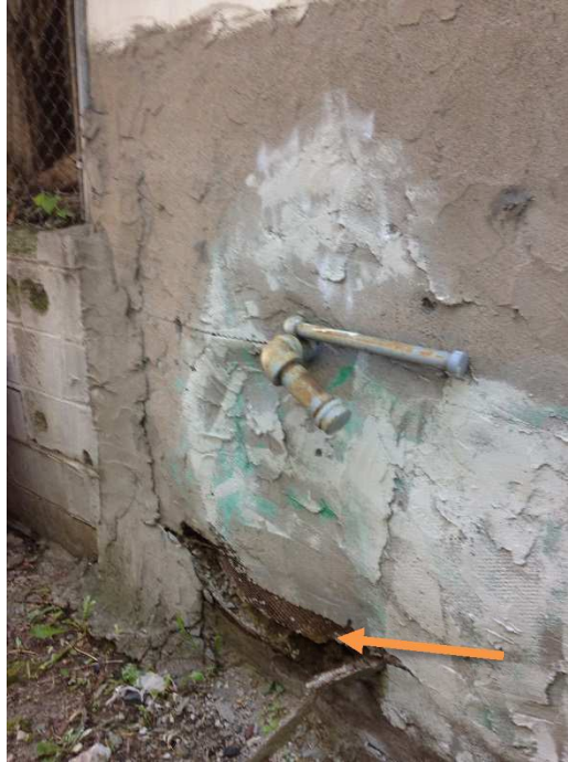
Picture 12 – Stucco Deterioration
