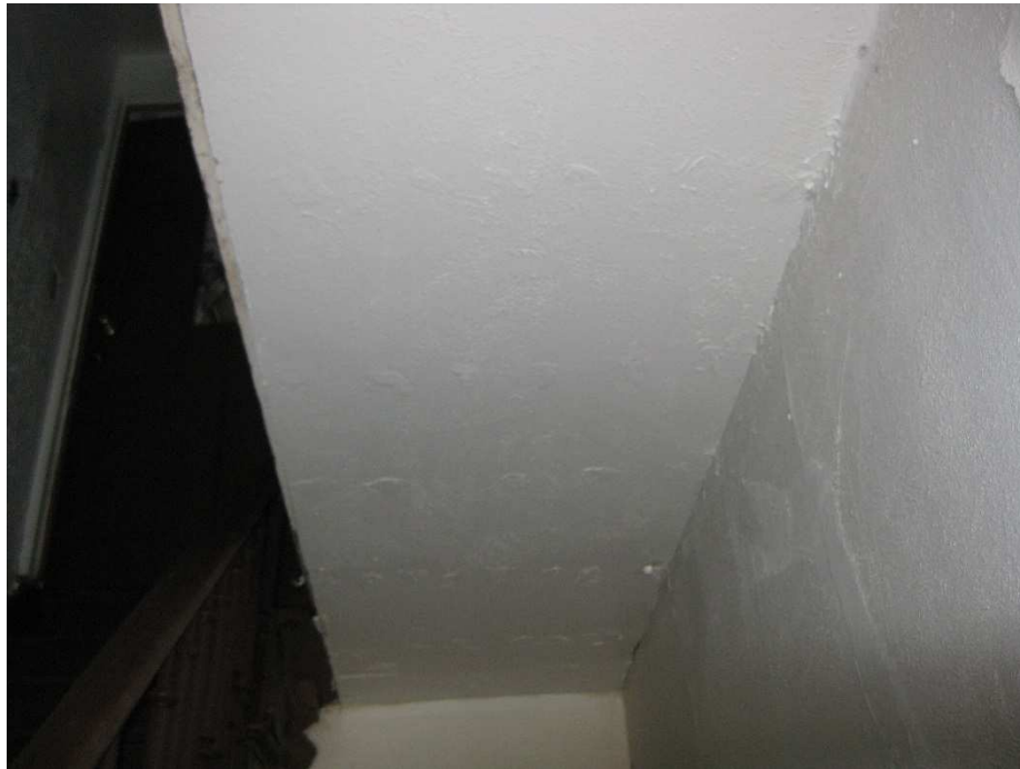
Picture 3 – Underside of Uneven Floor
