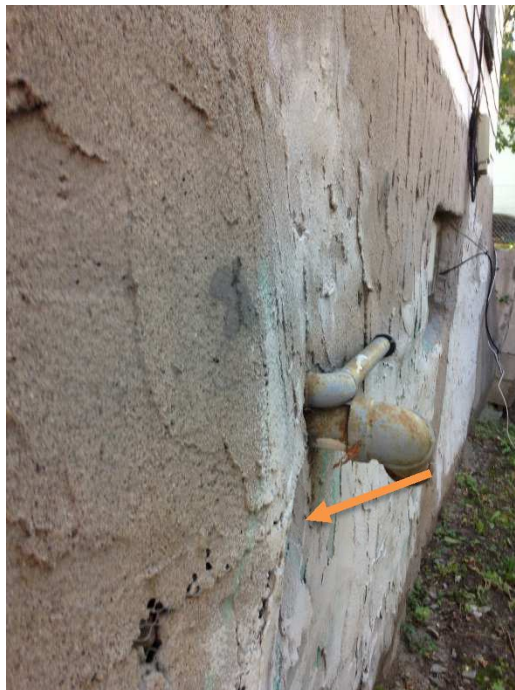
Picture 13 – Stucco Bulging Out
