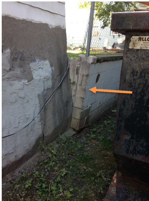
Picture 11 – Retaining Wall Out of Plumb
