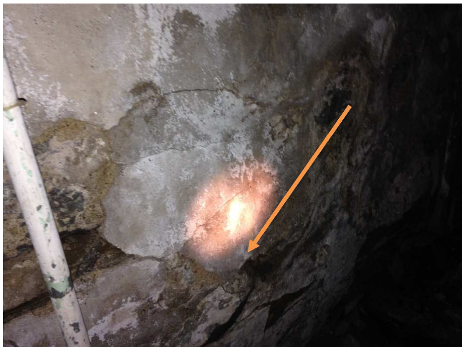
Picture 8 – Crumbling and Cracking of Foundation Walls
