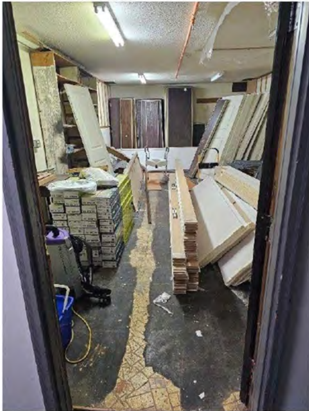
Photo 15 12" Yellow Floor Tile and Mastic in Damaged Condition in the 2 nd Floor East Employee Room.
