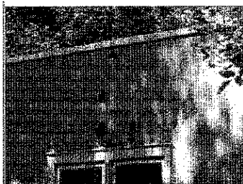
1 Exterior Wall Hazard
