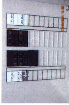
EXISTING T-MOBILE AC PANEL
