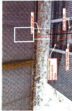
NEW ZAYO CABINET LOCATION
