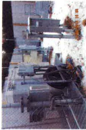
EXISTING T-MOBILE EQUIPMENT
