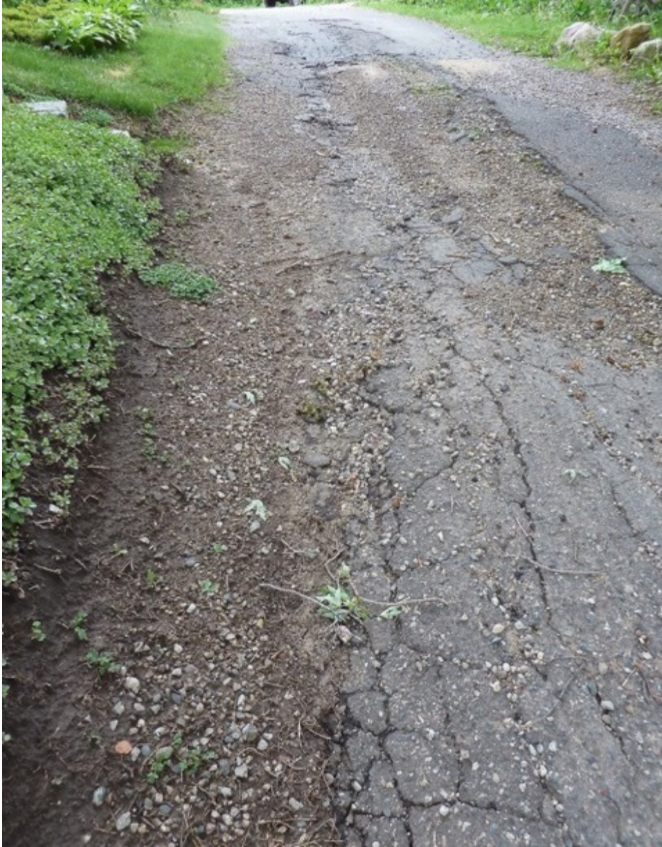
Photo 2. Erosion – North Side (May 2012)
