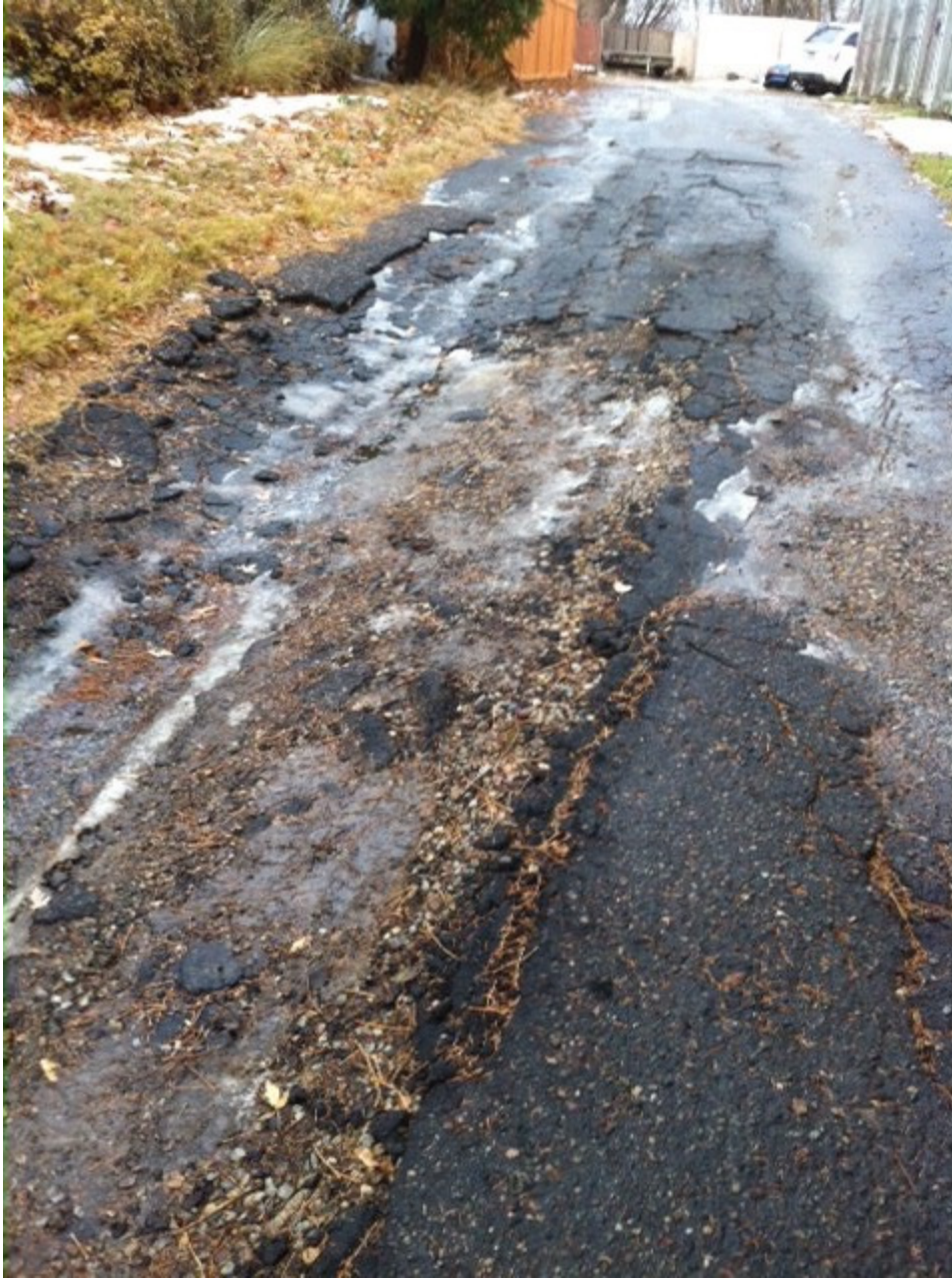
Photo 3. Same view as Photo 2, but taken Nov. 2014. Compare condition of pavement.
