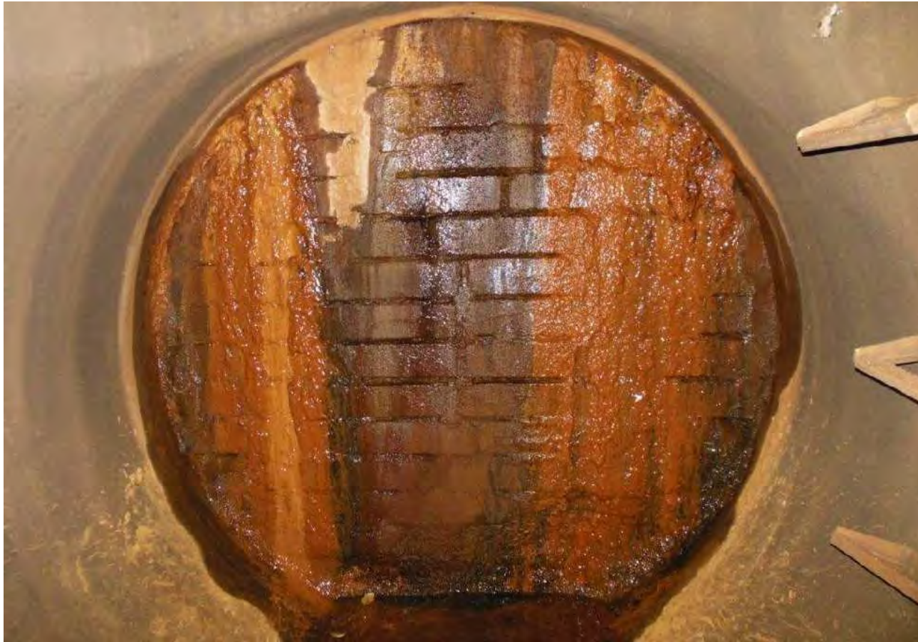
Iron Bacteria on Bulkhead
