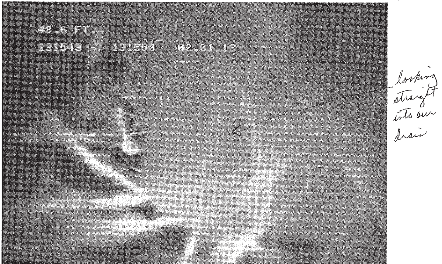
(camera shot looking into your private pipe; heavy roots)
