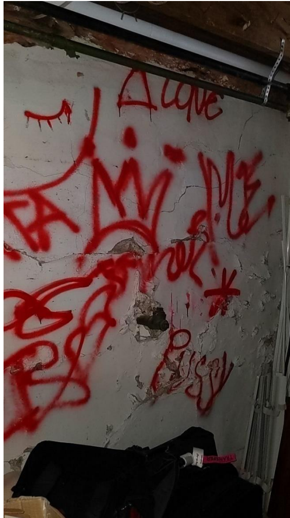
Figure 1: Parge Coating at End of Life (Delaminated)
